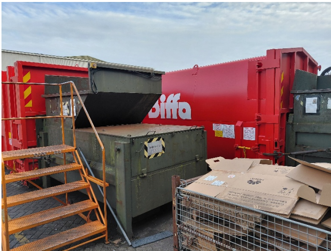
Photo 3. Two large compactors; one for general waste and one for cardboard.
