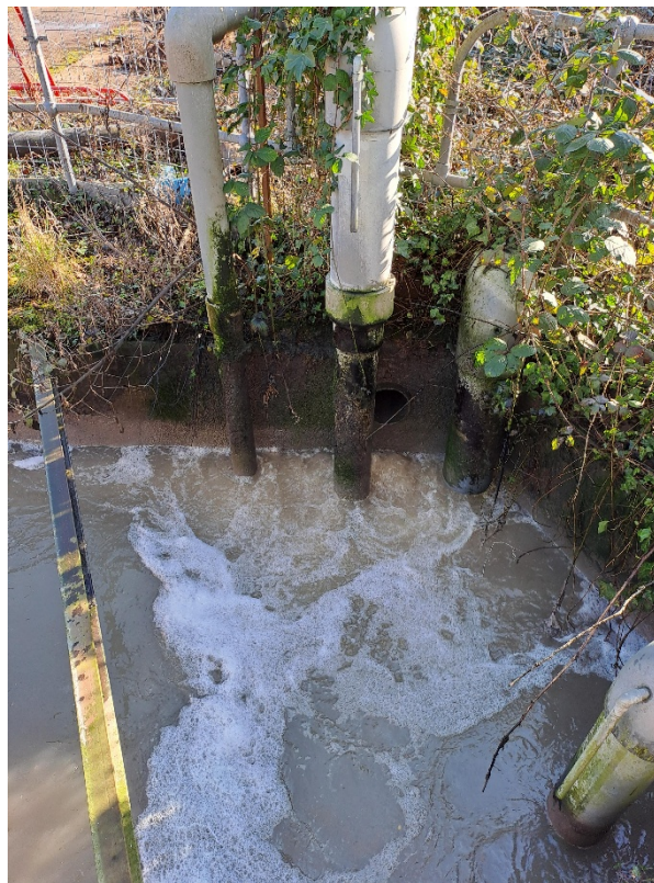
Figure 2 – The white pipe seen is where effluent discharge from Star Villas enters the treatment works without flow monitoring capturing the volume.
