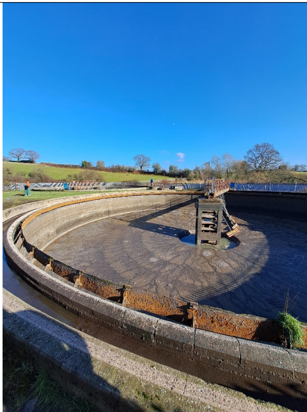
Figure 13 (Top) – Baffles of Tank 5 showing considerable rust and defects, but maintenance scheduled by DCWW to rectify.
