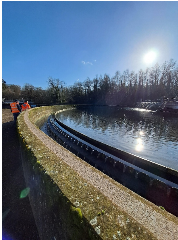
Figure 23 (Bottom) - Final Settlement Tank 4 as observed during the visit.
