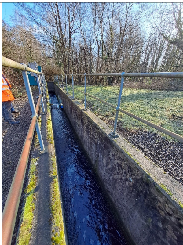
Figure 28 (Top) – Final effluent channel with monitors in situ.
