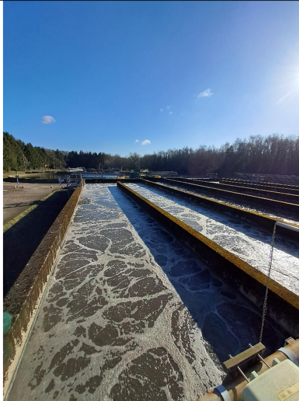
Figure 17 – The aeration lanes as observed during the visit
