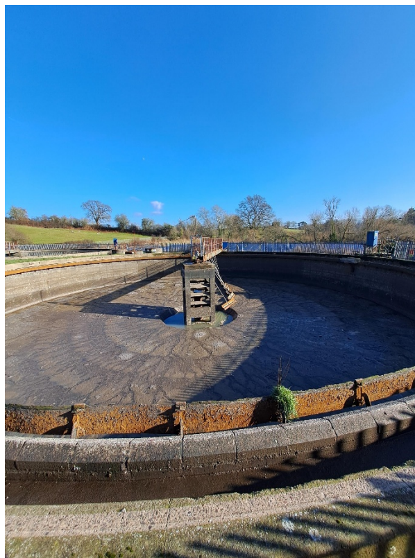
Figure 14 (Bottom) - Baffles of Tank 5 showing considerable rust and defects, but maintenance scheduled by
