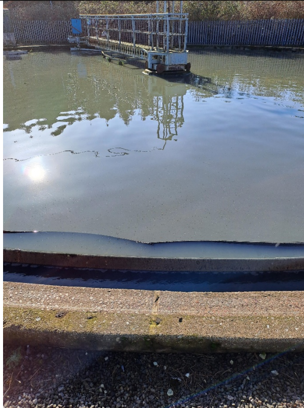
Figure 8 (Bottom) – A section of Settlement Tank 2's baffle where it has collapsed.
