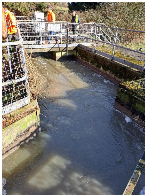
Figure 1 – The effluent as it enters the primary treatment site at the time of the visit.
