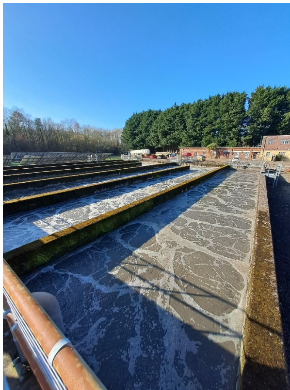
Figure 18 – The aeration lanes as observed during the visit.
