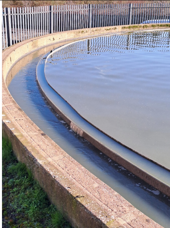
Figure 10 (Top): Settlement tank 4 baffle breach as observed during the visit.
