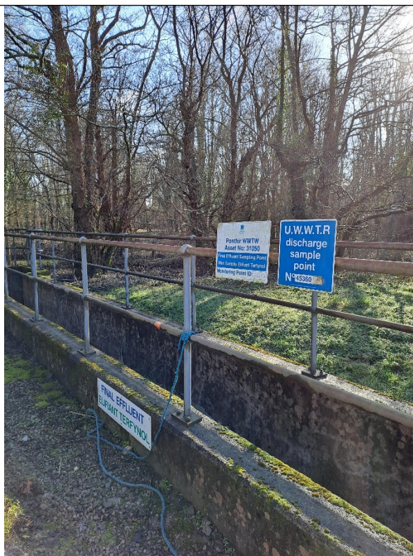
Figure 25 (Top) - The final effluent sampling point, clearly labelled.
