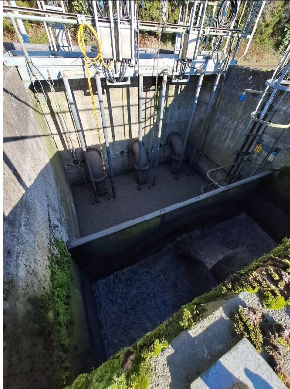
Figure 24 – The sludge return system as observed during the visit.
