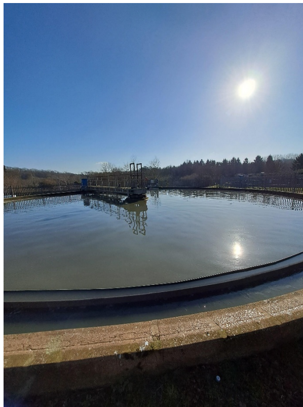
Figure 11 (Bottom): General condition of Settlement tank 4 as observed during the visit.
