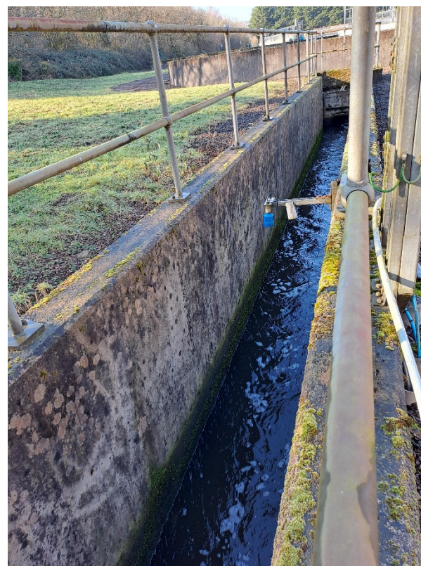
Figure 29 (Bottom) – Final effluent channel with monitors in situ.
