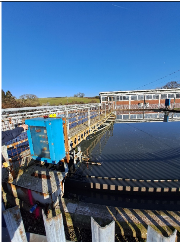
Figure 5 (Top) – Settlement tank 1 where the metal plate restricting the bridge rotation can be seen on the chamber wall.
