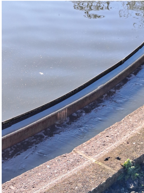
Figure 7 (Top) – Settlement Tank 2's scum board overtopping.
