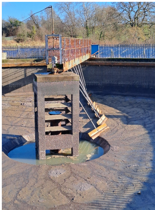
Figure 12 – Settlement Tank 5 drained down for maintenance at the time of the visit.
