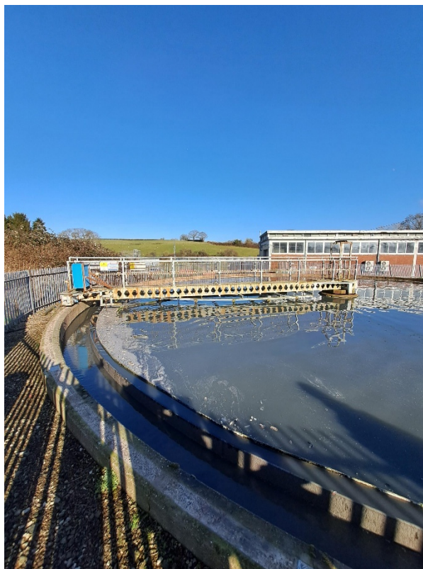
Figure 6 (Bottom) – The general condition of Settlement tank 1 at the time of the visit.
