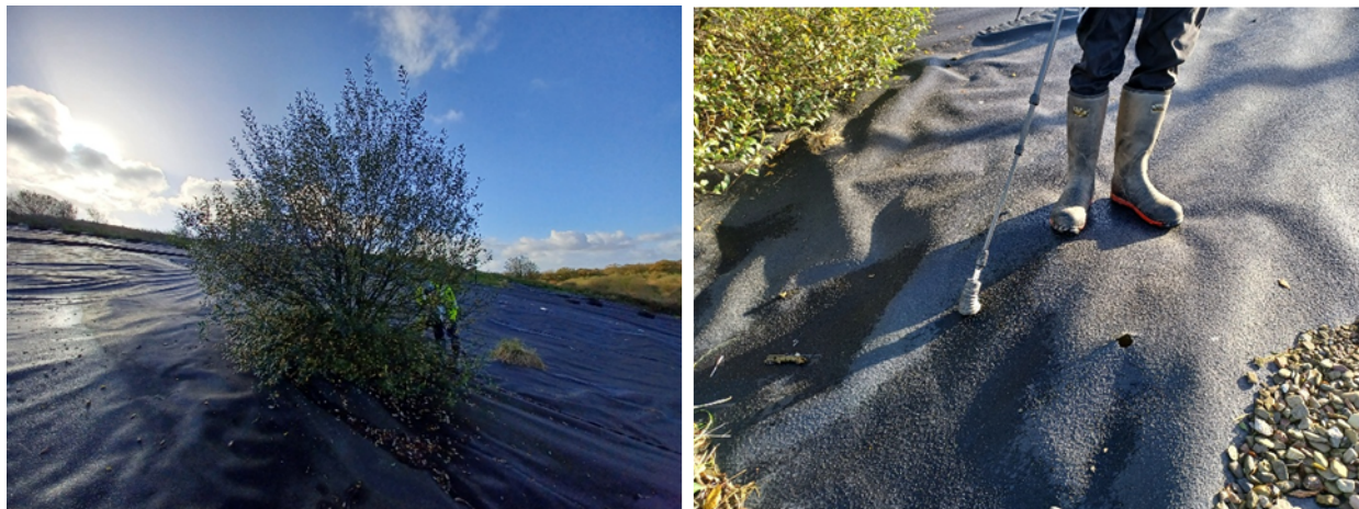
Images 3 & 4: Examples of observed failures on the Landfill Cap
