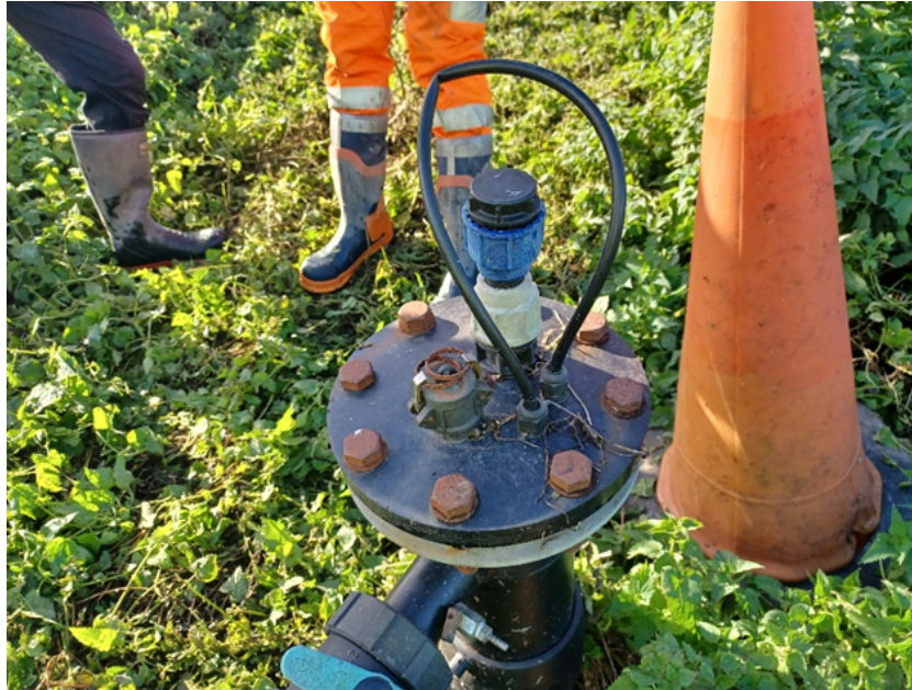
Image 2: Loss of Landfill Gas from redundant cable coupling points associated with NYCL0013
