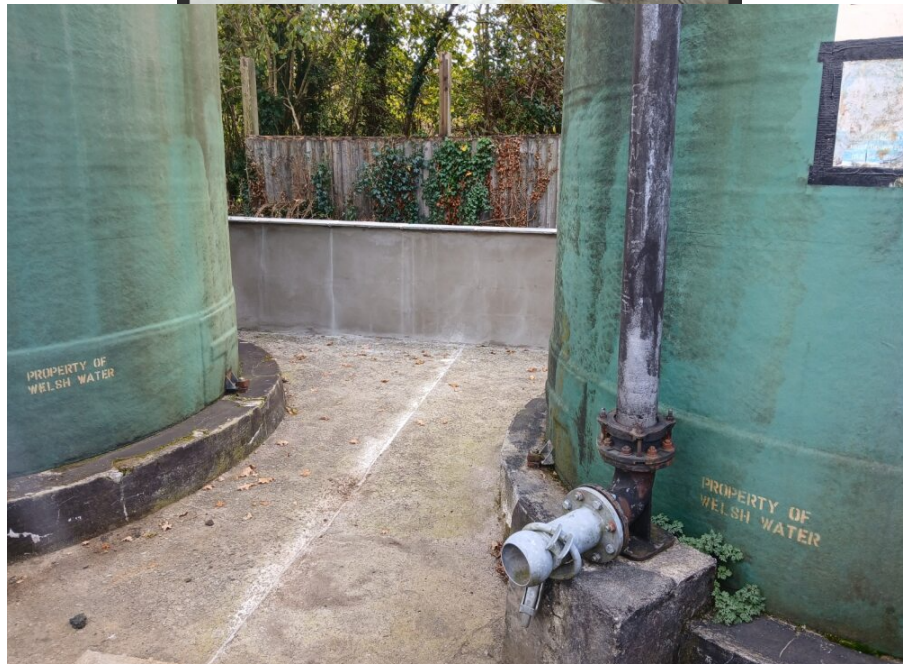
Annex 2- Tertiary Containment
