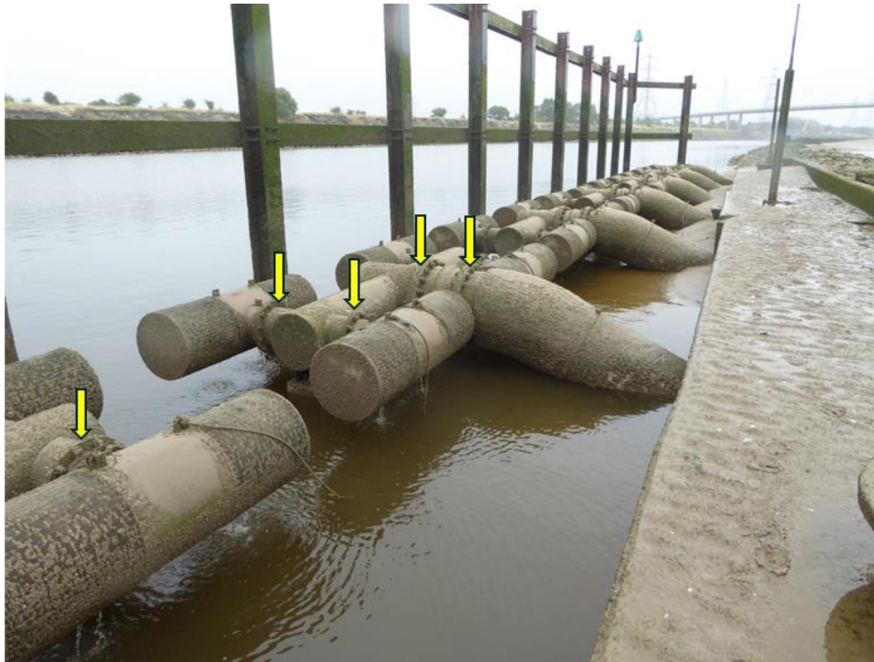
Figure 6: Eel Screens at the Water Connection Corridor
