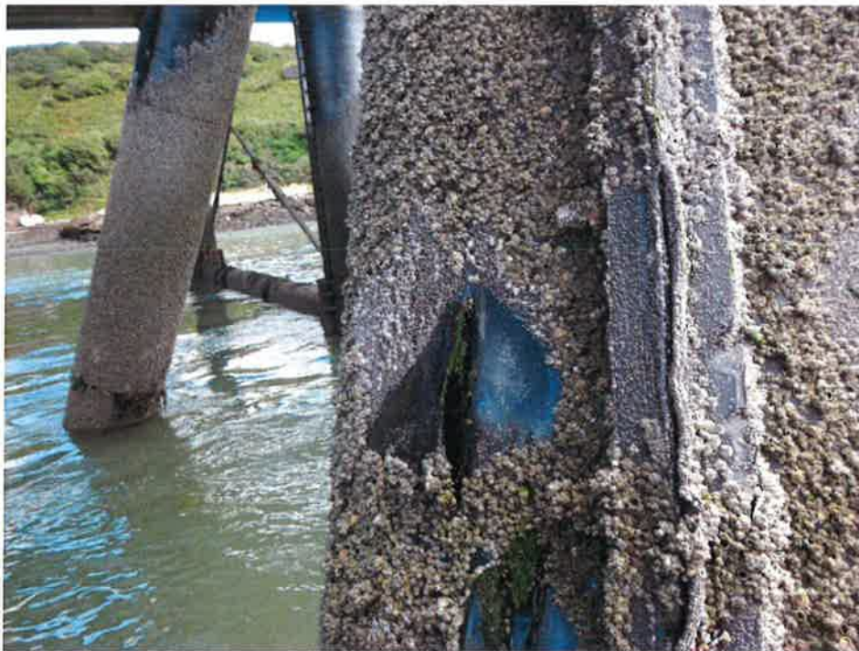
Figure 11: EMD6 Sea Shield damage - Remove, inspect and renew
