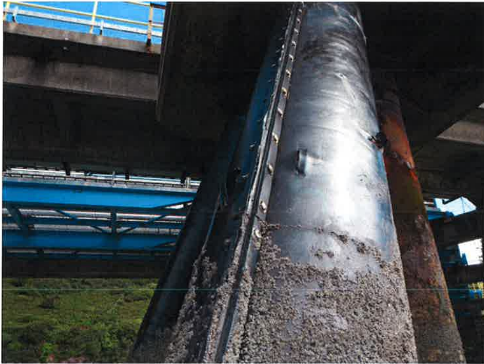
Figure 10: EMD6 Sea Shield damage - Remove, inspect and renew
