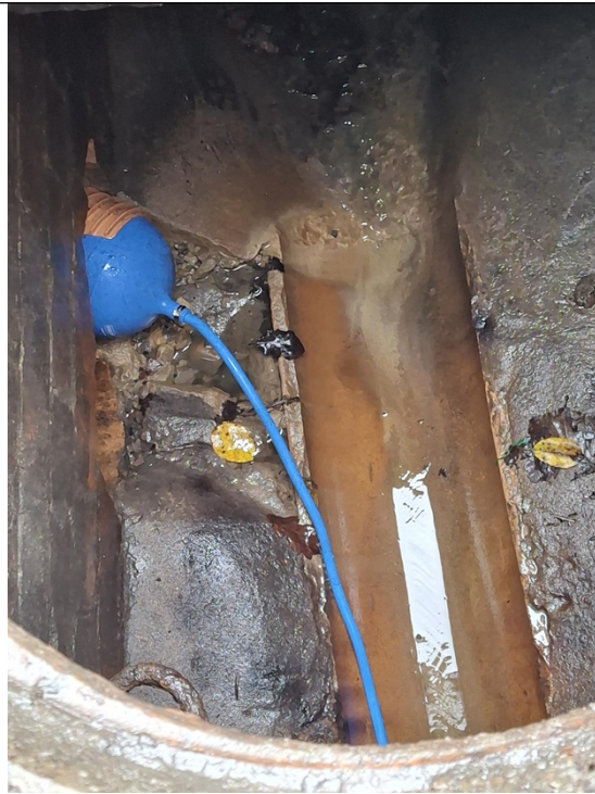
Fig 3: Bund in place in private surface water line where TW had connected
