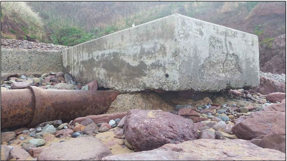
PHOTO B - UNDERMINING OF MANHOLE CONCRETE SURROUND (TAKEN 17/10/16)
