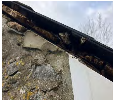
Photograph 4 showing potential bat roosting features on building (TN6).
