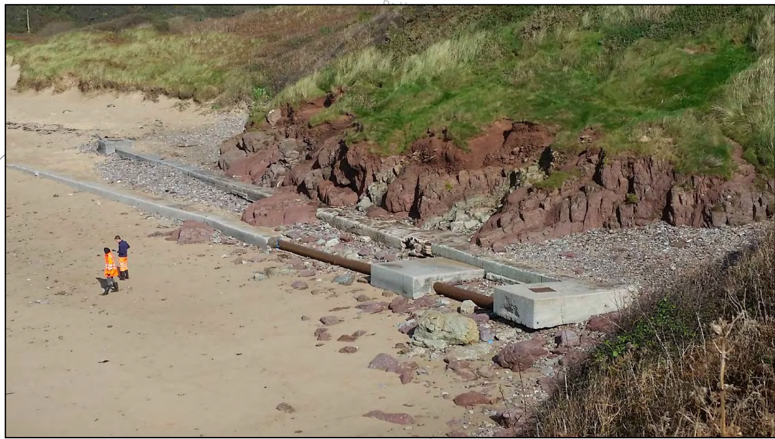
PHOTO A - EXPOSED PIPE SECTIONS AT TOP OF BEACH (TAKEN 17/10/16)
