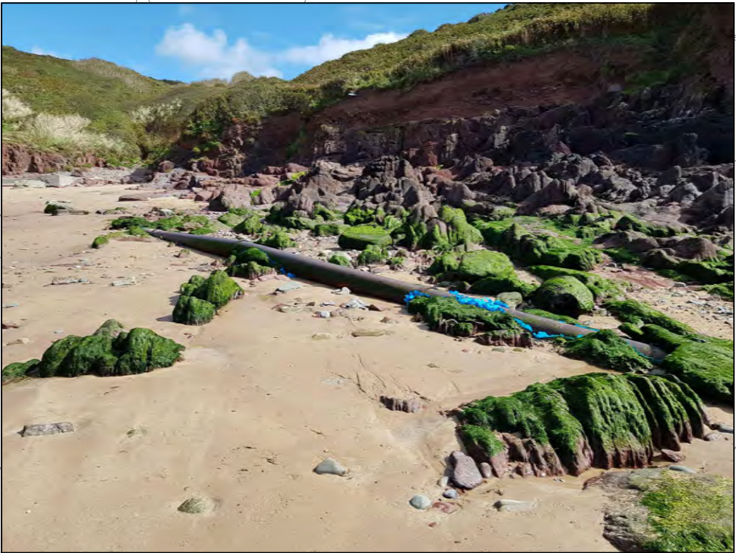
PHOTO C - EXPOSED PIPE SECTION PART WAY DOWN BEACH (TAKEN 13/09/18)
