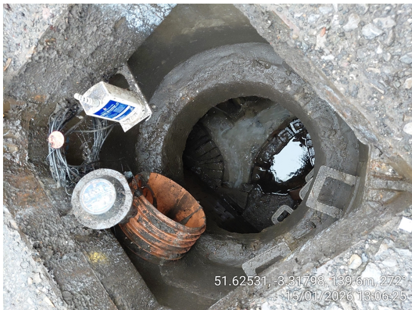
Image 1: CSO chamber. Orange overflow pipe.
