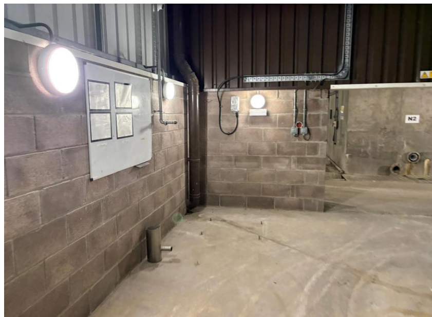
Figure 2: Millenium Farm Compressor Area
