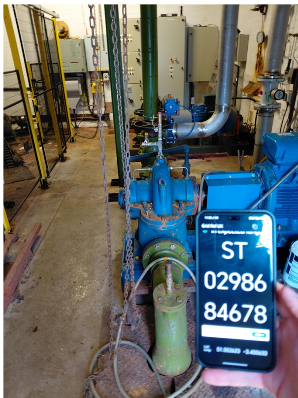
Photograph 1: Abstraction location in pump room
