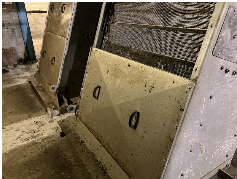
Photograph 2: Storm and settled storm screens
