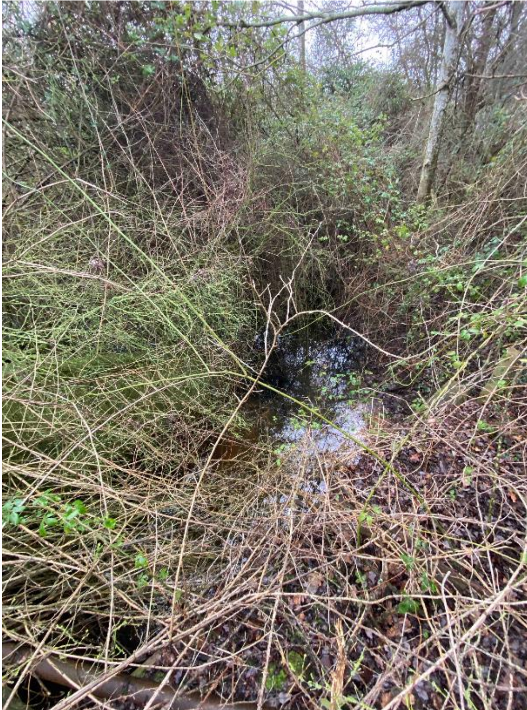
Photograph 10: Location 08: Talacre Brook meandering south due to concrete construction walls diverting it underneath a road via another culvert with a pipe (diameter 1.8m). The brook is ~6.5m wide and ~2.5m deep at this point. Photo taken facing north.
