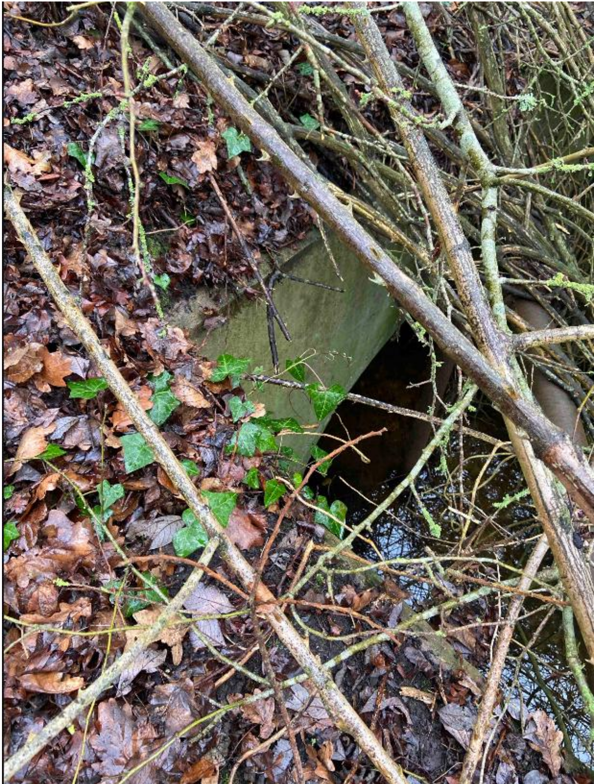
Photograph 11: Location 08: Previously mentioned in Photograph 10, this is the second culvert, which is 1.8m diameter.
