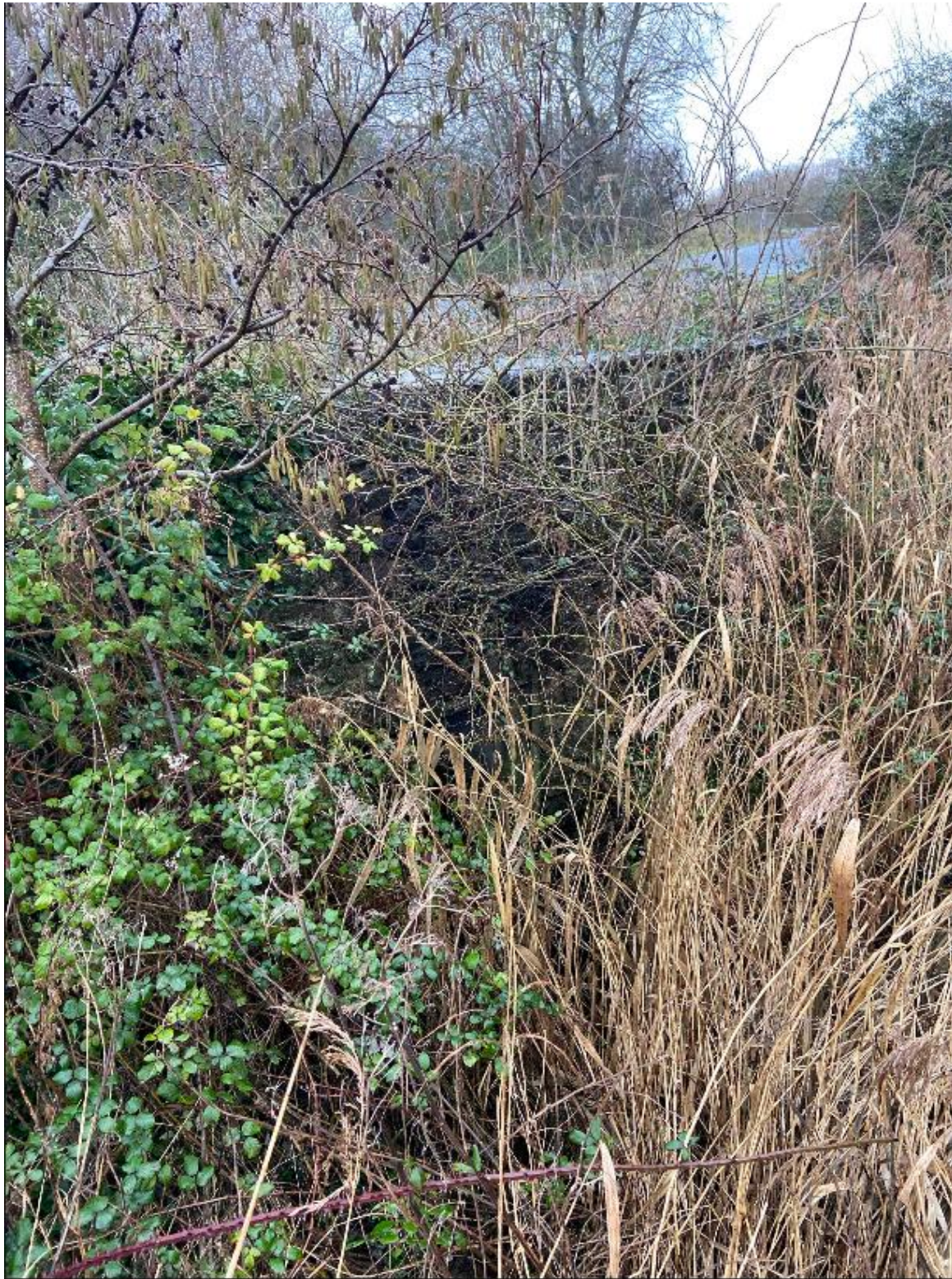
Photograph 9: Location 07: Cobblestone culvert underneath historic road. The culvert is a pipe with a diameter of 0.7m. At this point Talacre brook is ~6.0m wide and ~2.0m deep with a low flow present. Difficult to photograph as heavy vegetation completely surrounding. Photo taken facing east.
