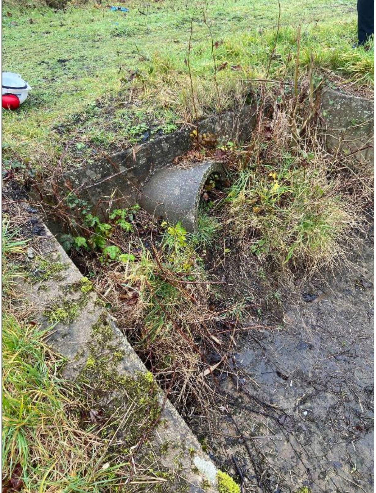
Photograph 19: Location 12: Discharge pipe for Talacre Brook, pipe 0.5m diameter. Covered with vegetation but still very slow flow visible.
