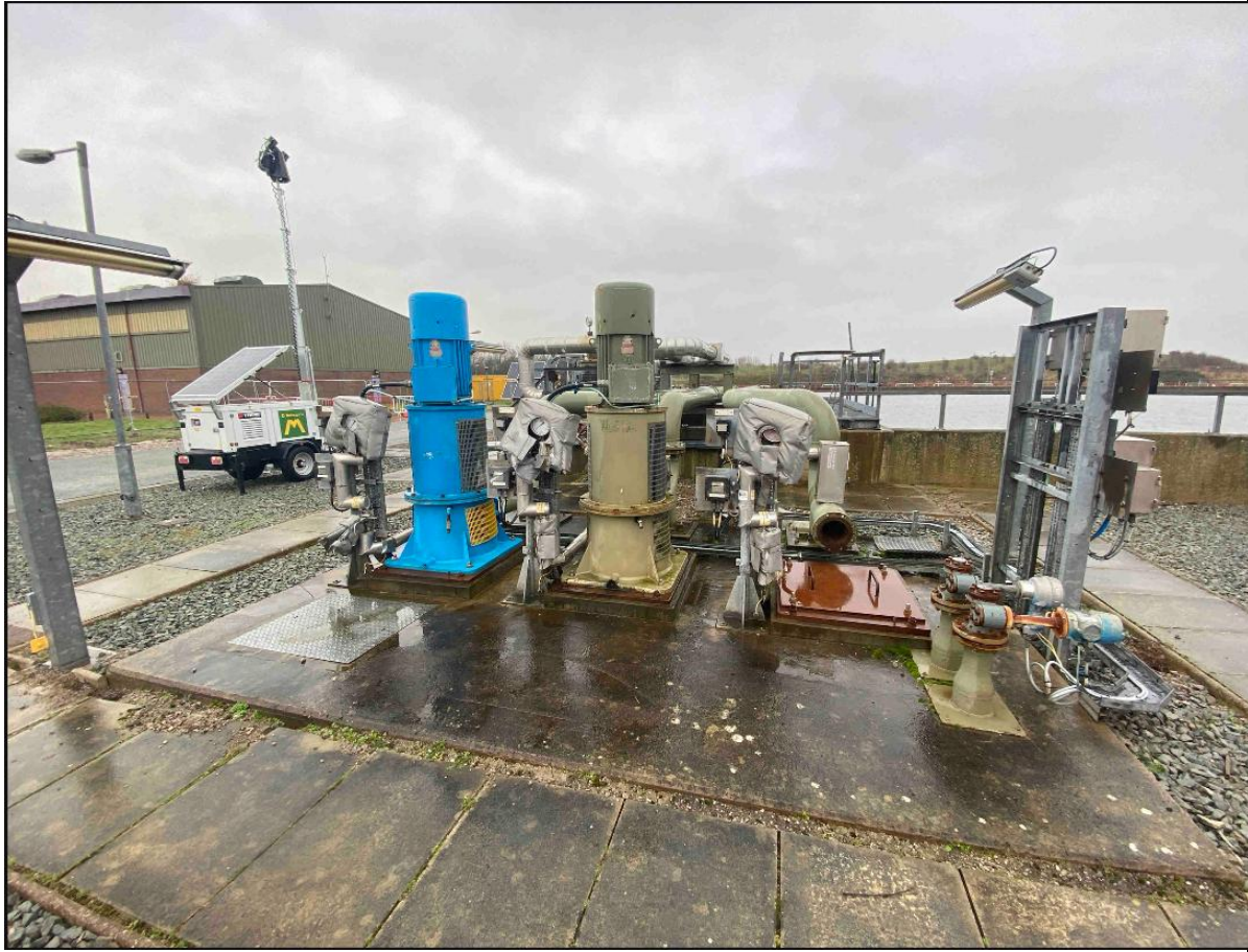
Photograph 2: Location 00: Permanent installation pumps on site for the surface water storage tank (Maximum capacity of 50m 3 per hour)
