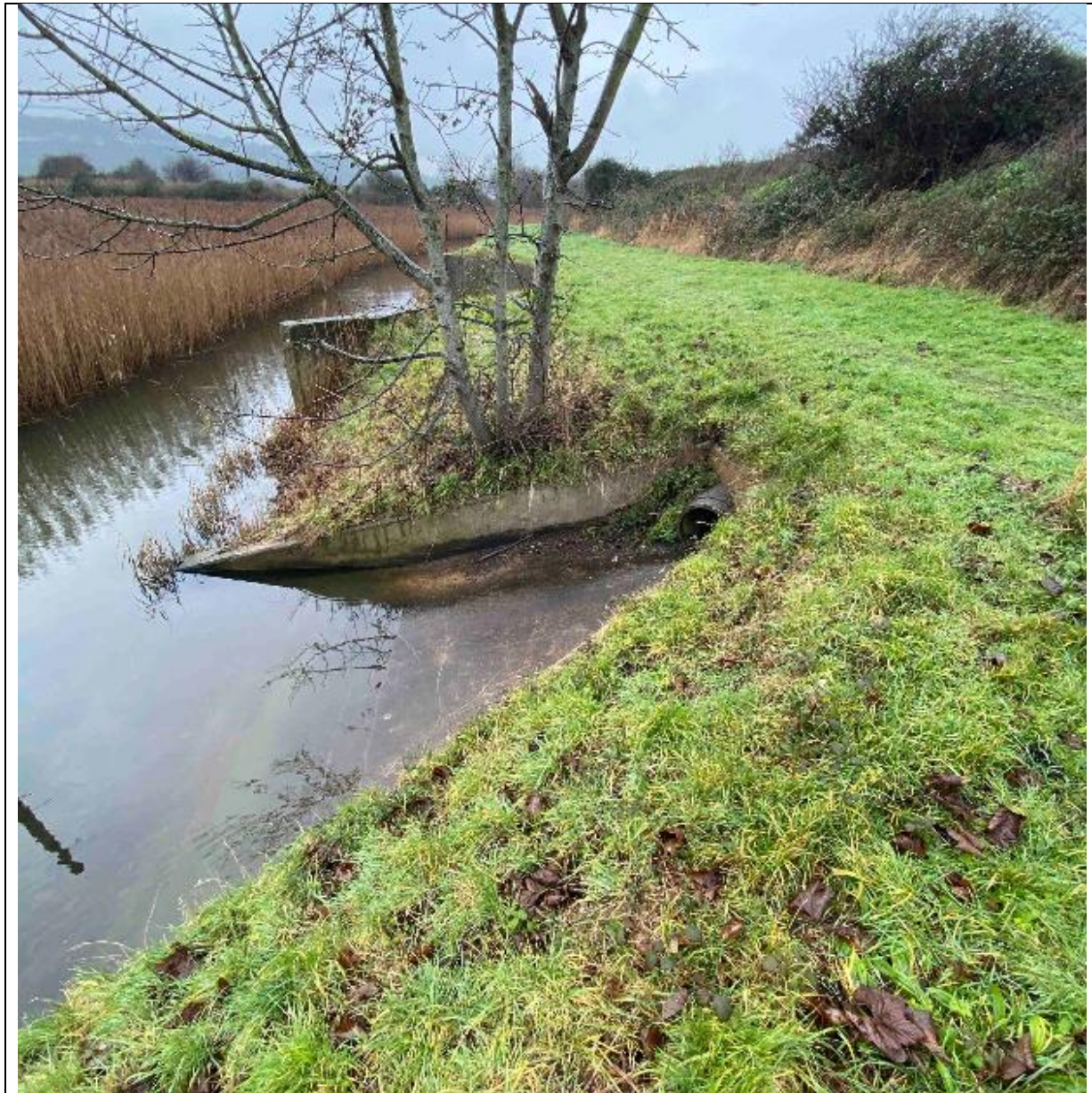
Photograph 16: Location 11: Discharge pipe outflowing to the lagoon, 450mm diameter pipe. No flow visible.
