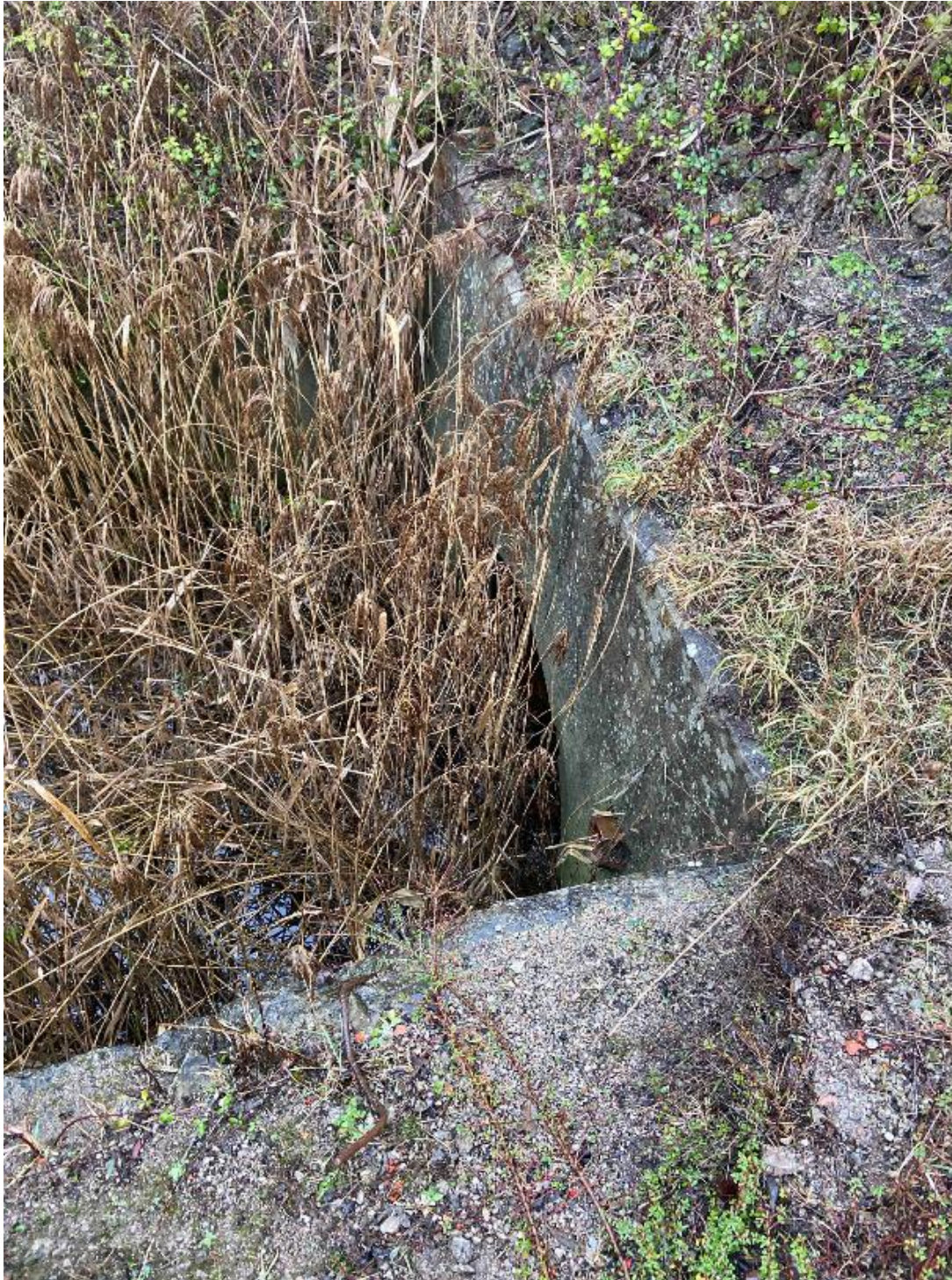
Photograph 12: Location 09: Outfall from culvert in Photograph 11, still with a diameter of 1.8m. The brook is built into a concrete channel here with a width of ~4.0m and a depth of ~2.5m. The brook then is directed into a drainage pipe that travels entirely underneath the old colliery, this pipe has a diameter of 1.5m at this entrance.
