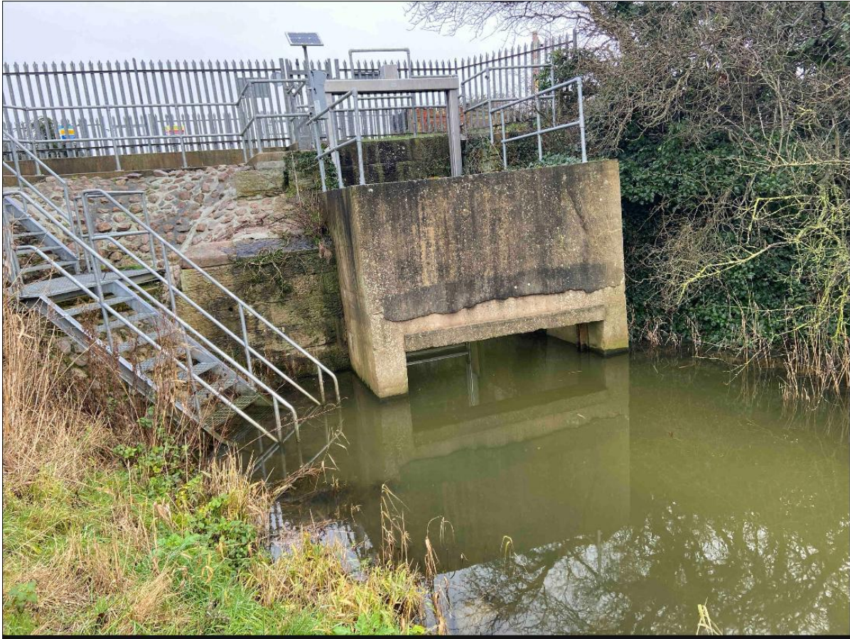
Photograph 15: Location 10: View of the sluice gate from the banks of the lagoon. Photo taken facing East.
