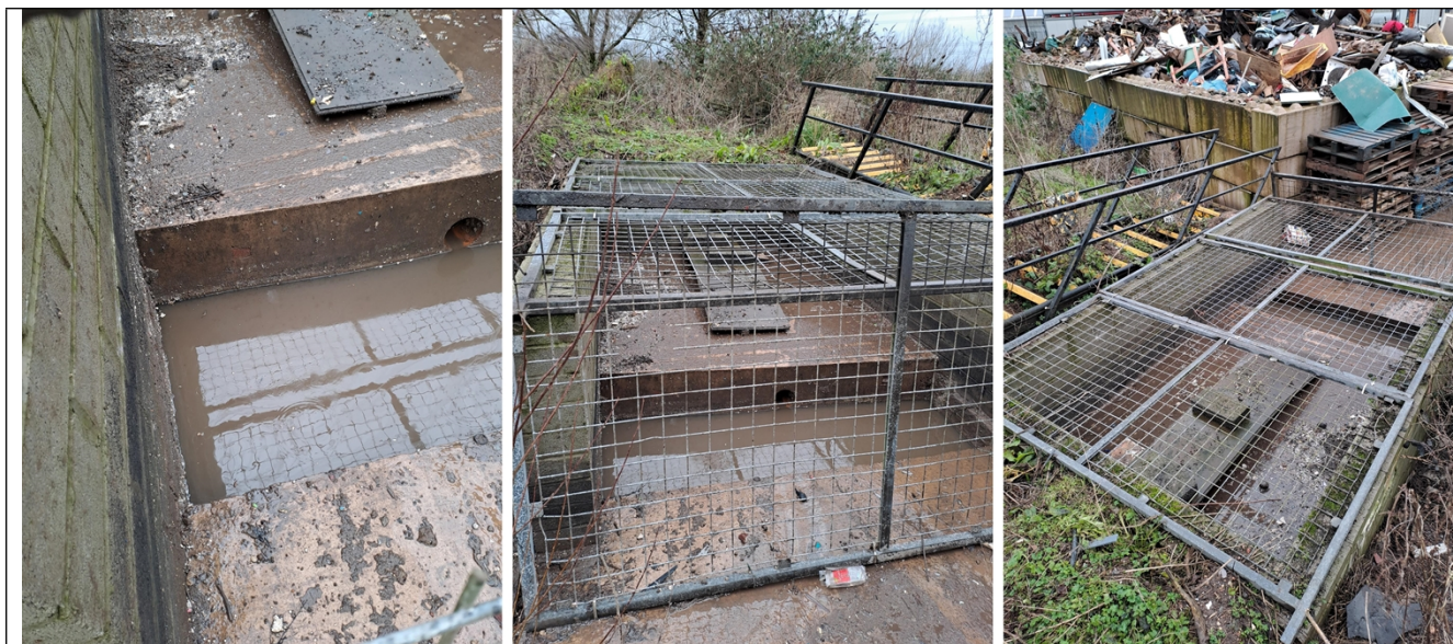
Figure 2 – The condition of the interceptor as observed during the visit.
