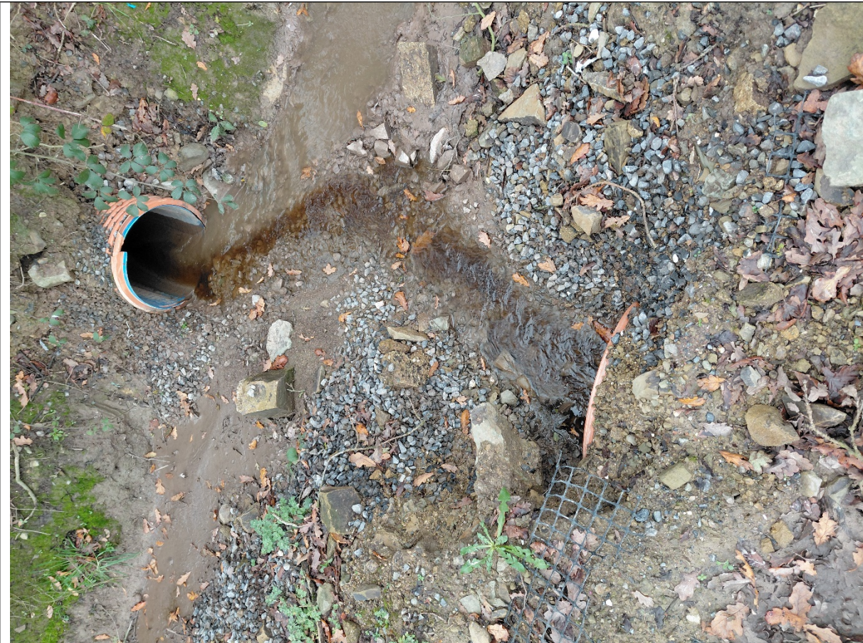
Figure 6 Photo showing unknown liquid discharging into open stream.
