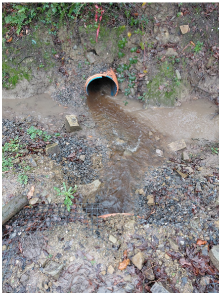
Figure 7 Photo above showing dark brown/black liquid emerging from pipe adjacent to compost leachate lagoon.
