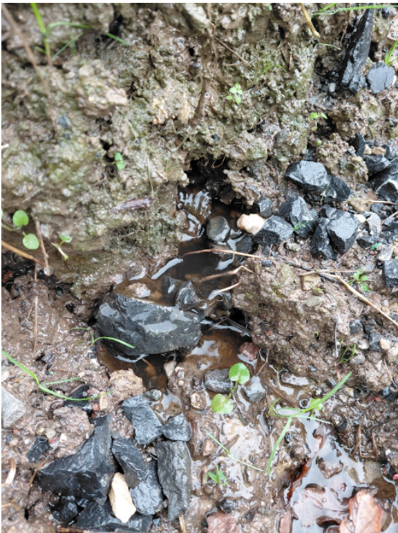
Figure 11 Photo above shows dark brown/black liquid flowing through leachate lagoon containment.
