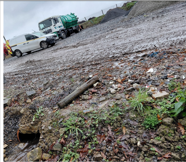
Figure 8 Photo above showing pipe appears to run from direction of compost leachate lagoon showing in the background.
