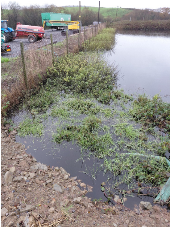
Figure 9 Photo above shows very high level of dark brown/black liquid in leachate lagoon.
