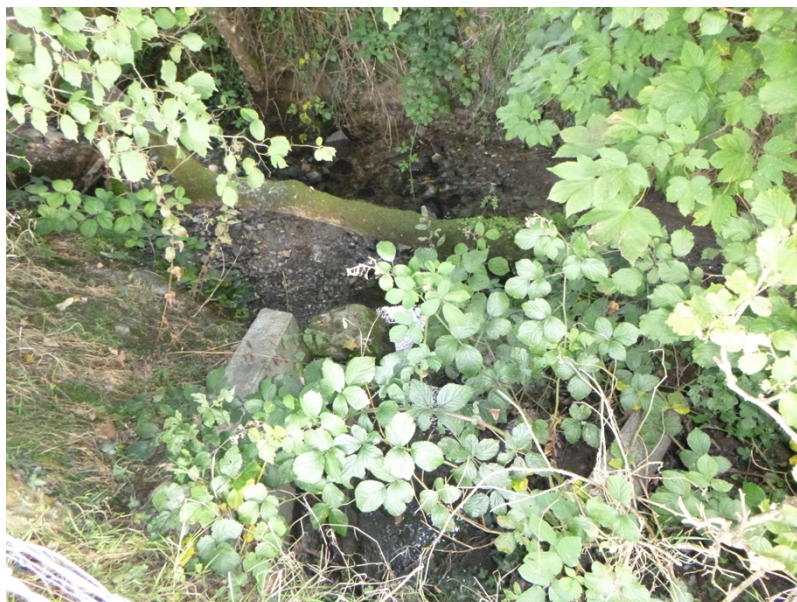
Photograph 4: Final effluent outfall
