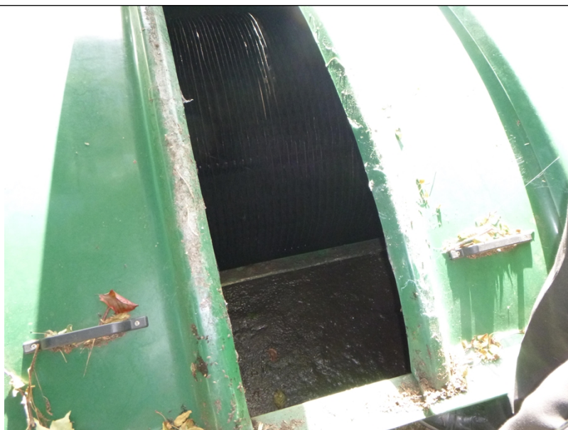
Photograph 2: Rotating Biological Contractor (RBC) discs
