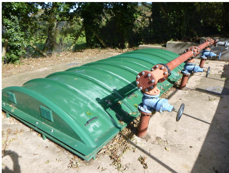
Photograph 1: Rotating Biological Contractor (RBC)
