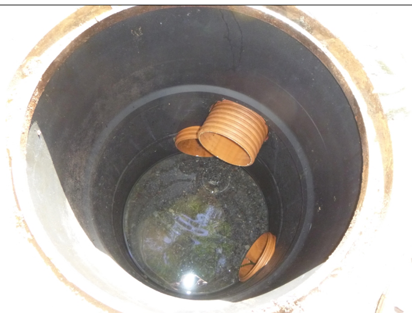
Photograph 3: Final effluent sample point
