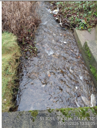
Image 2. Downstream of the point of discharge of the CSO, Nant Gwawr, NGR SO 01087 01725
