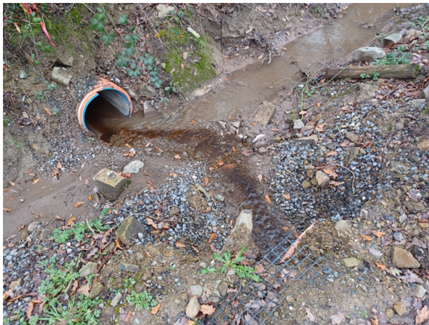
Image 1: Evidence of a discoloured discharge believed to be entering the surface water network associated with the Phase 2 Landfill
