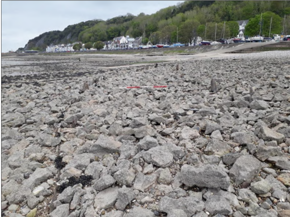
Plate 30. Remains of wooden groyne/jetty 05799w and slipway 057998w. Note sewage pipe ion the background. View to the south-southeast, scale in 0.5m divisions.
