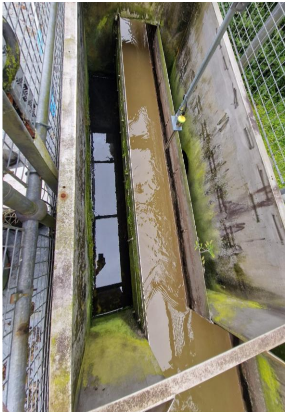
Storm Overflow Weir
