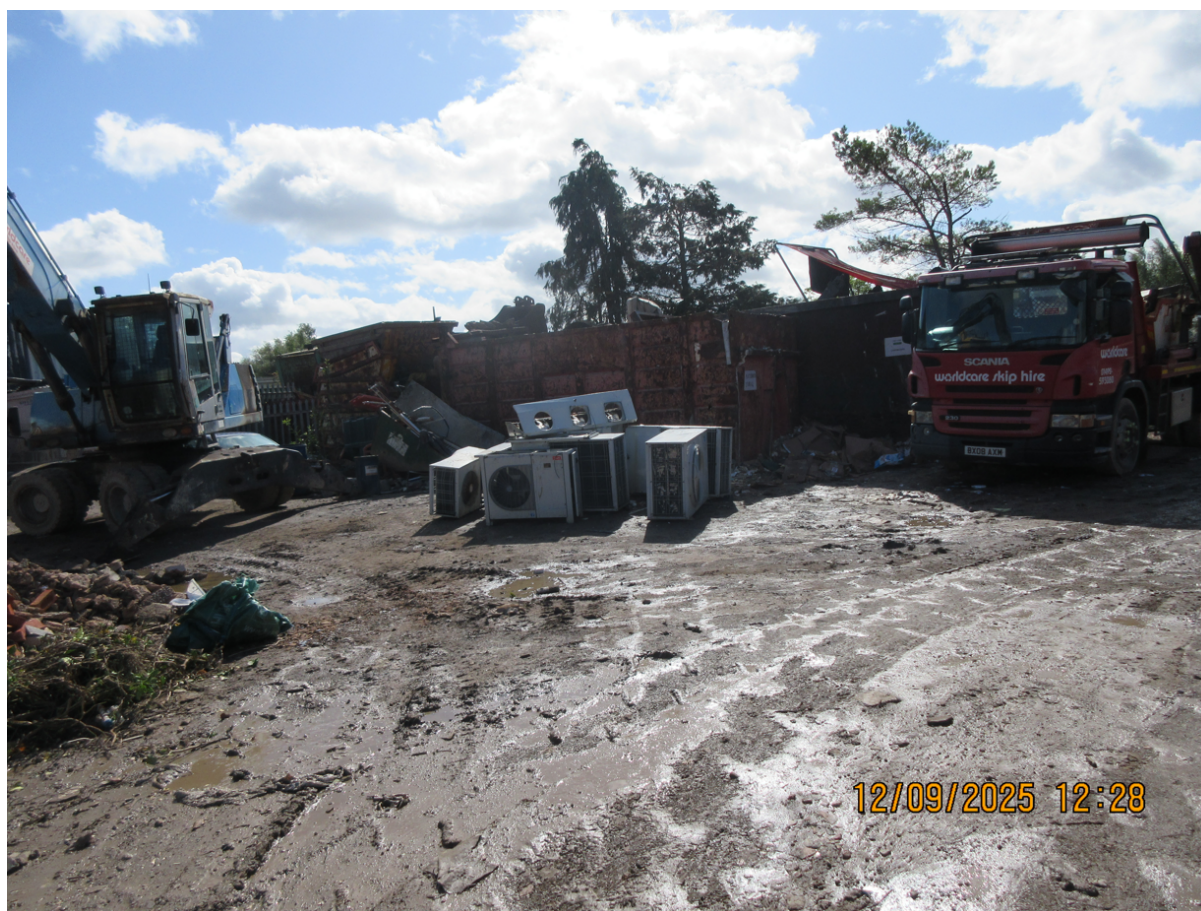
Photograph 3, non-permitted air conditioning units
