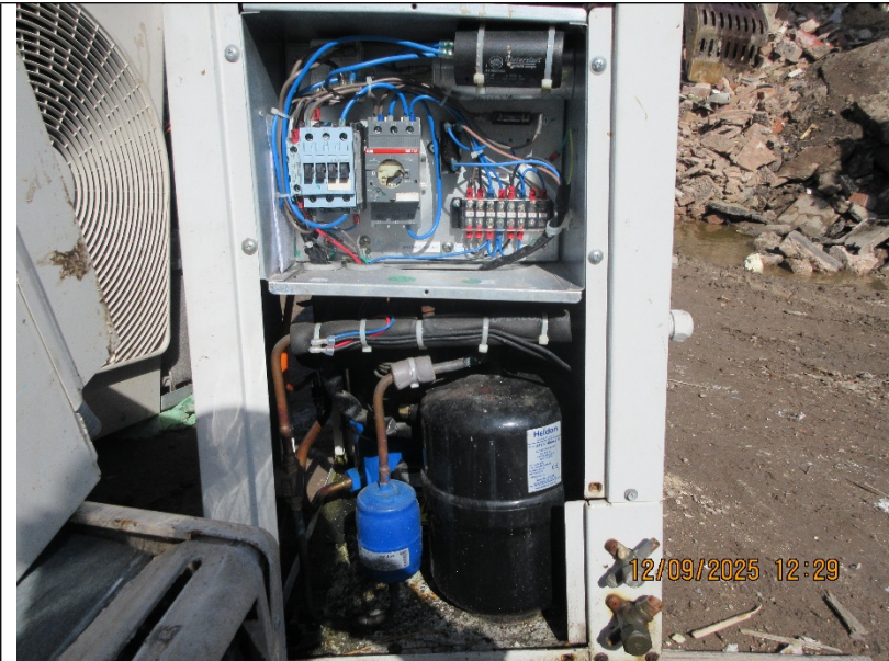
Photograph 2 - Internal components of the air conditioning units.
