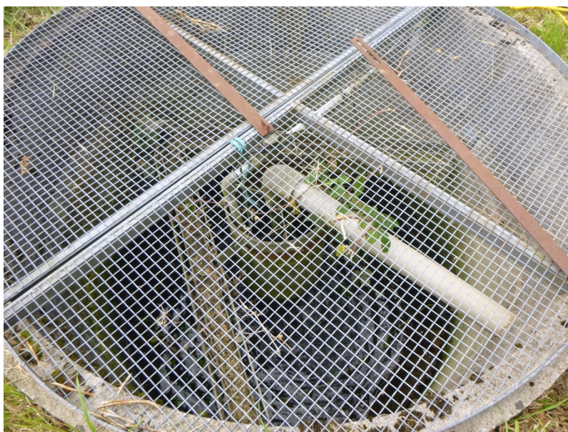
Photograph 4: Post-filter bed chamber
