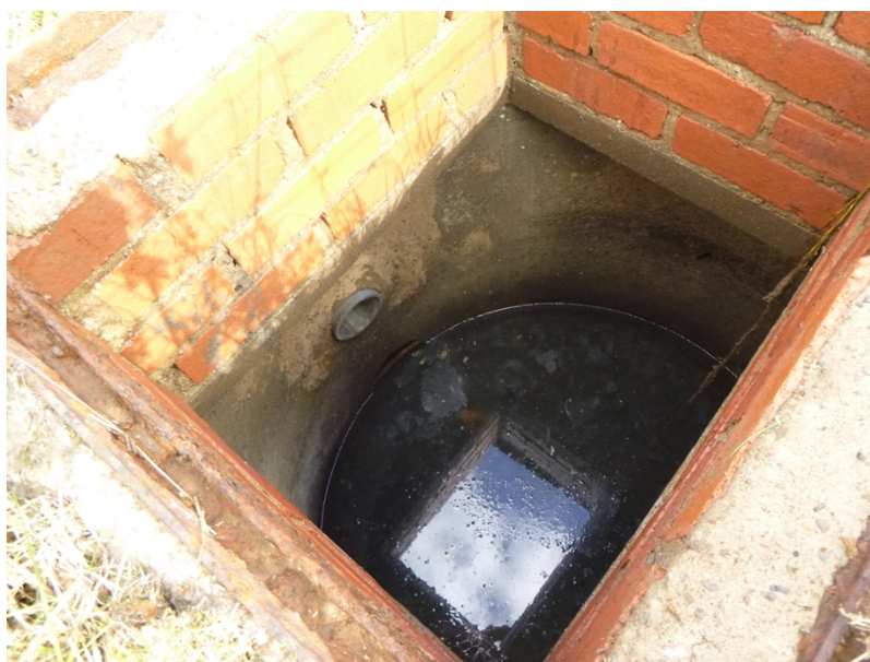
Photograph 6: Final effluent sample point
