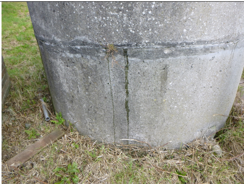
Photograph 3: Leak in filter bed wall
