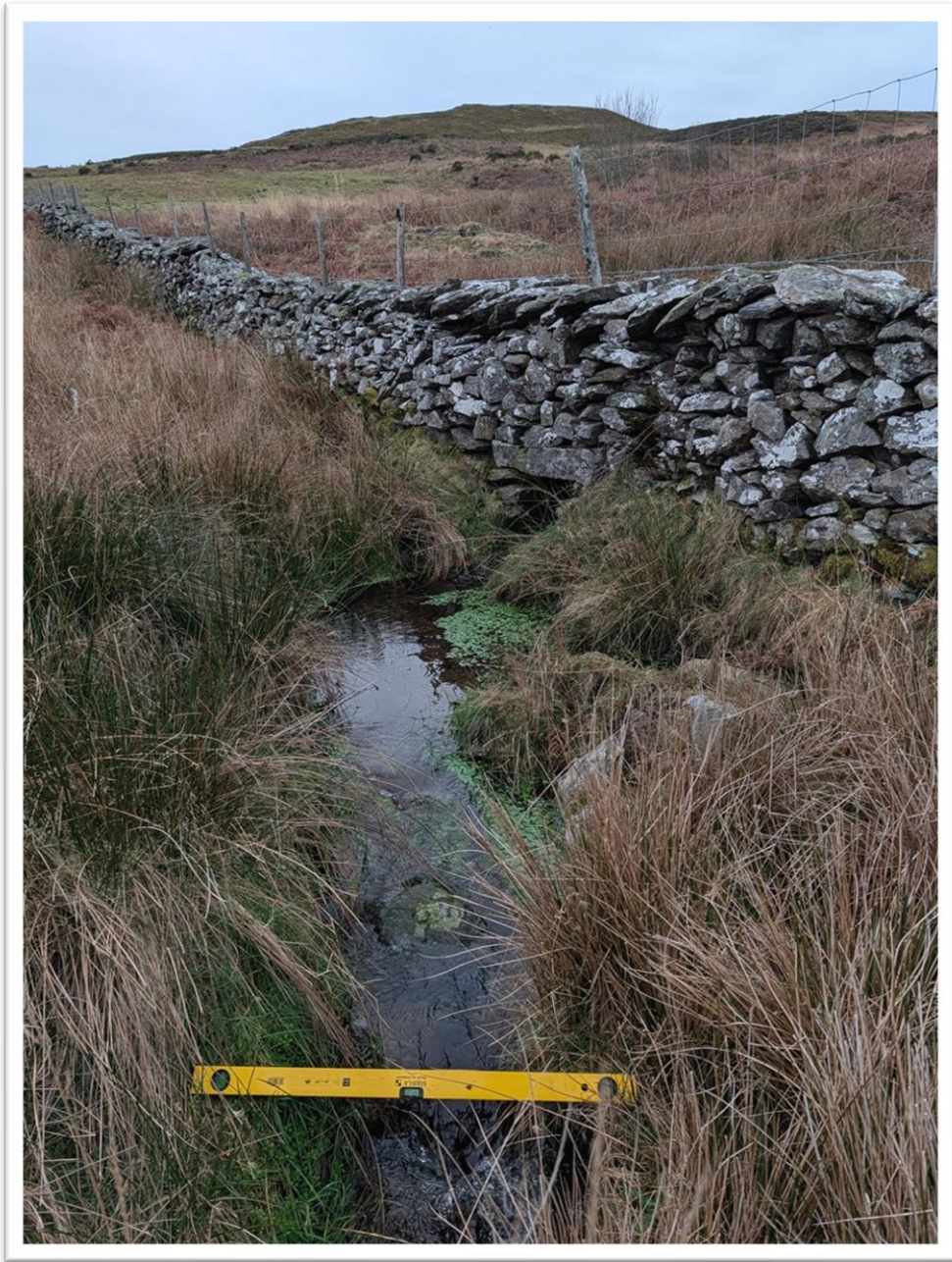
Photos taken both sides of wall. Looking upstream from downstream side of the wall.
