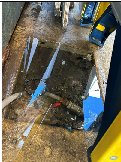
Image 10. Sump to the rear of the bund which is filled with silt and plastic debris.
