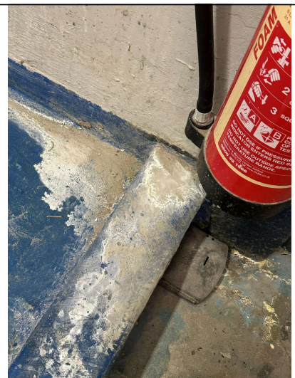
Image 14. Heavy chemical staining within / outside the bund and on top of the bund walls.
