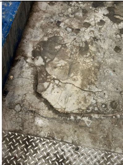
Image 10. Heavy chemical staining and damage to the warehouse floor. Many cracks visible.
