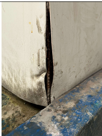
Image 13. Delamination of the tank decorative outer skin.
