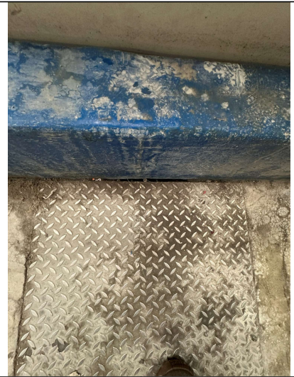
Image 8. Internal drainage channel running beneath the bunded area.
