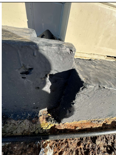
Image 11. Historic evidence of vehicular impact.
