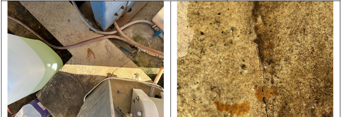
Image 4. Damage to the bund wall adjacent to the dewatering system. Image 5. Cracks to the bund floor are visible throughout the structure.
