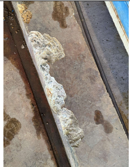
Image 8. Damage to the bund wall from forklift impact (suspected wheels when turning).
