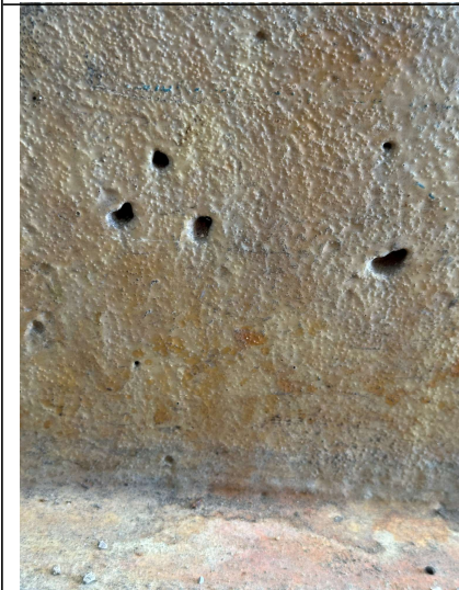
Image 12. Pitting / holes observed to the lining of the bund walls.
