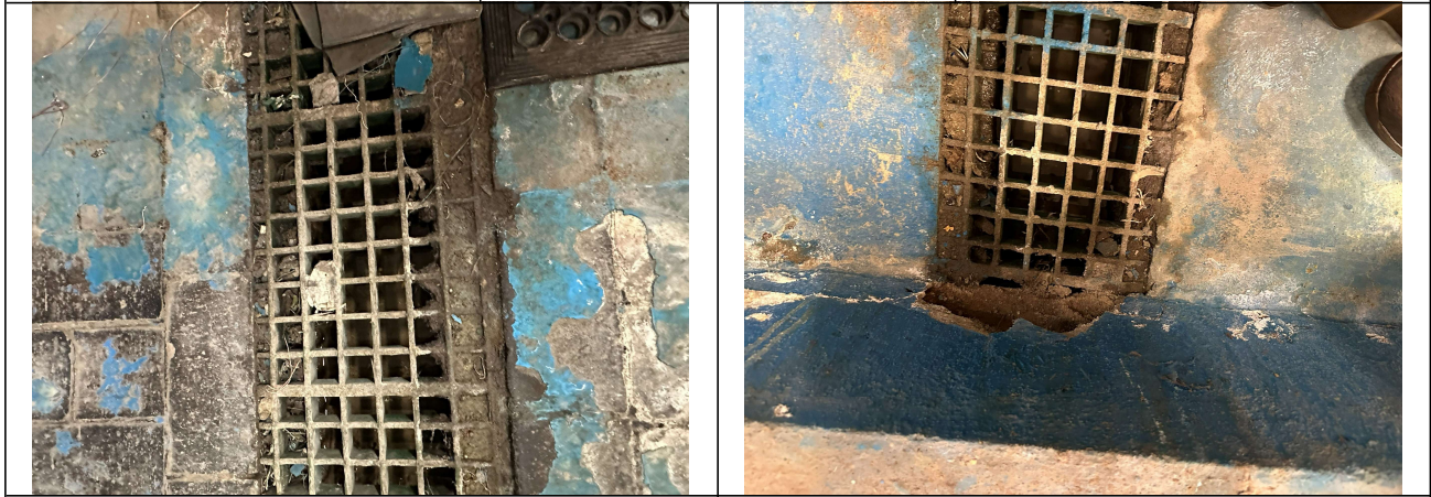
Image 4. Drainage channel passing through the warehouse floor and discharging to bund 2 (externally). Image 5. Drainage channel passing through the warehouse floor and discharging to bund 2 (externally).
