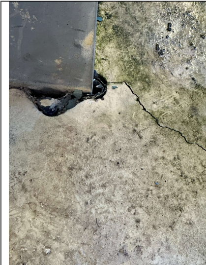
Image 6. Cracks to the bund wall to the rear of the concrete structure (rear, right hand side).
