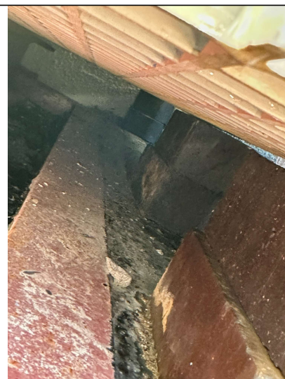
Image 12. Ancillary equipment held above the bunded area on bricks and plastic gratings.
