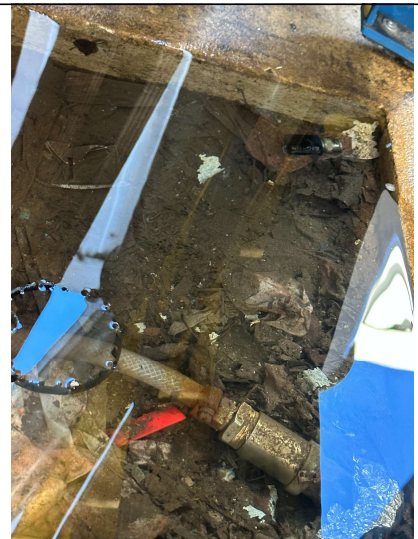
Image 11. Sump to the rear of the bund which is filled with silt and plastic debris.
