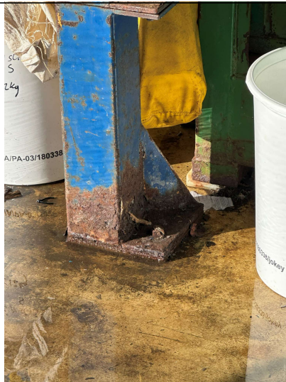
Image 13. Corroded steel supports which were submerged in rainwater.
