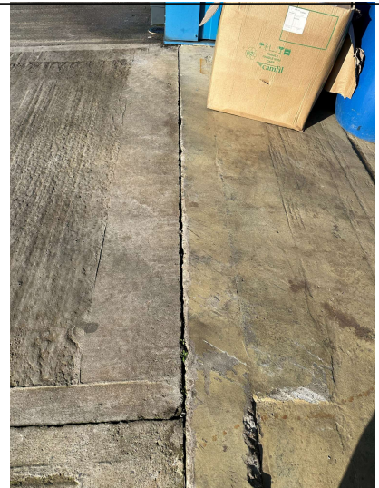
Image 14. Unsealed gap between the bund floor and the external concrete pad - pollutant pathway.
