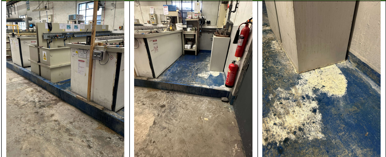
Image 1. View of the tanks held within the bunded area. Image 2. Storage area within the confines of the secondary containment. Image 3. Heavy chemical staining and corrosion noted to large areas of the bund.
