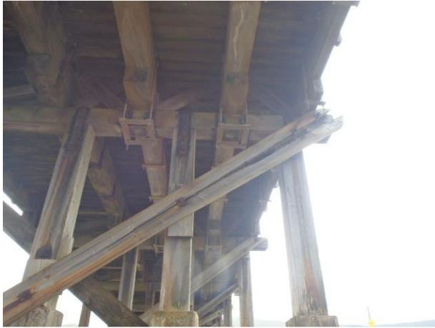
Timber beam to be replaced
