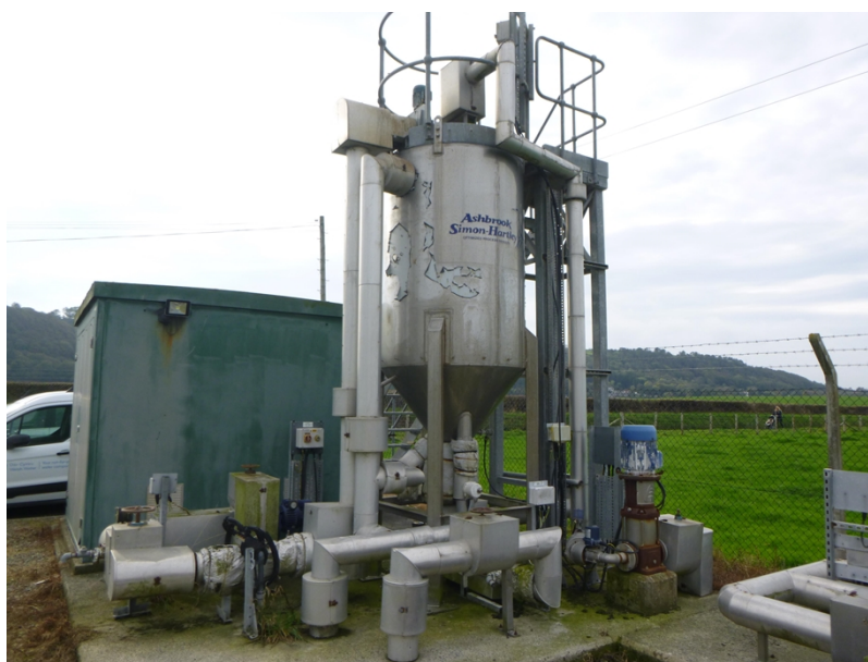
Photograph 10: Sludge treatment system
