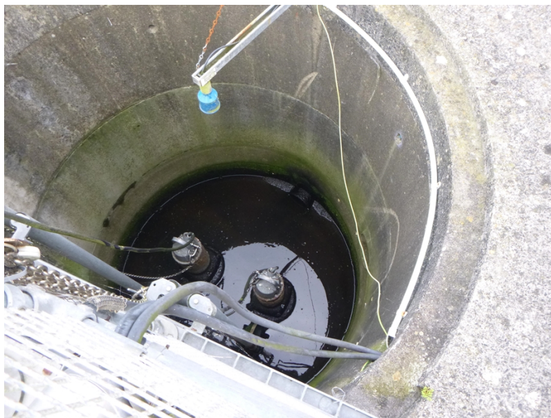
Photograph 8: Final effluent collection chamber
