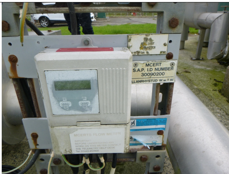
Photograph 9: MCERTS flow meter
