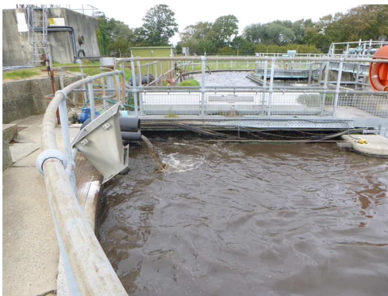
Photograph 4: Aeration ditch and activated sludge return pipe
