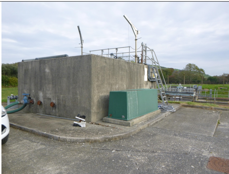
Photograph 11: Sludge holding tank
