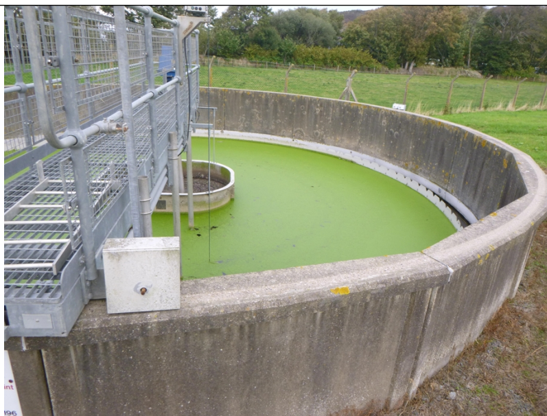
Photograph 5: Final settlement tank
