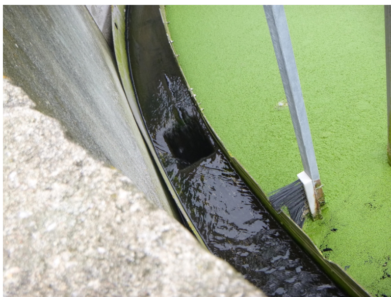
Photograph 6: Final effluent sample point
