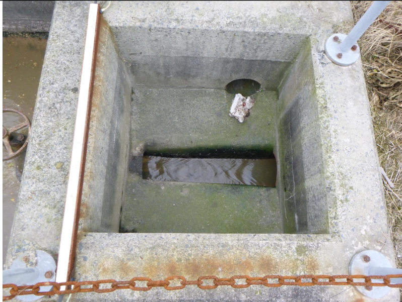
Photograph 1: Storm overflow at gravity inlet
