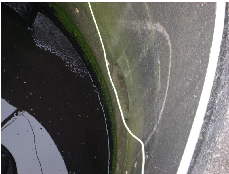
Photograph 3: Emergency overflow within final effluent chamber
