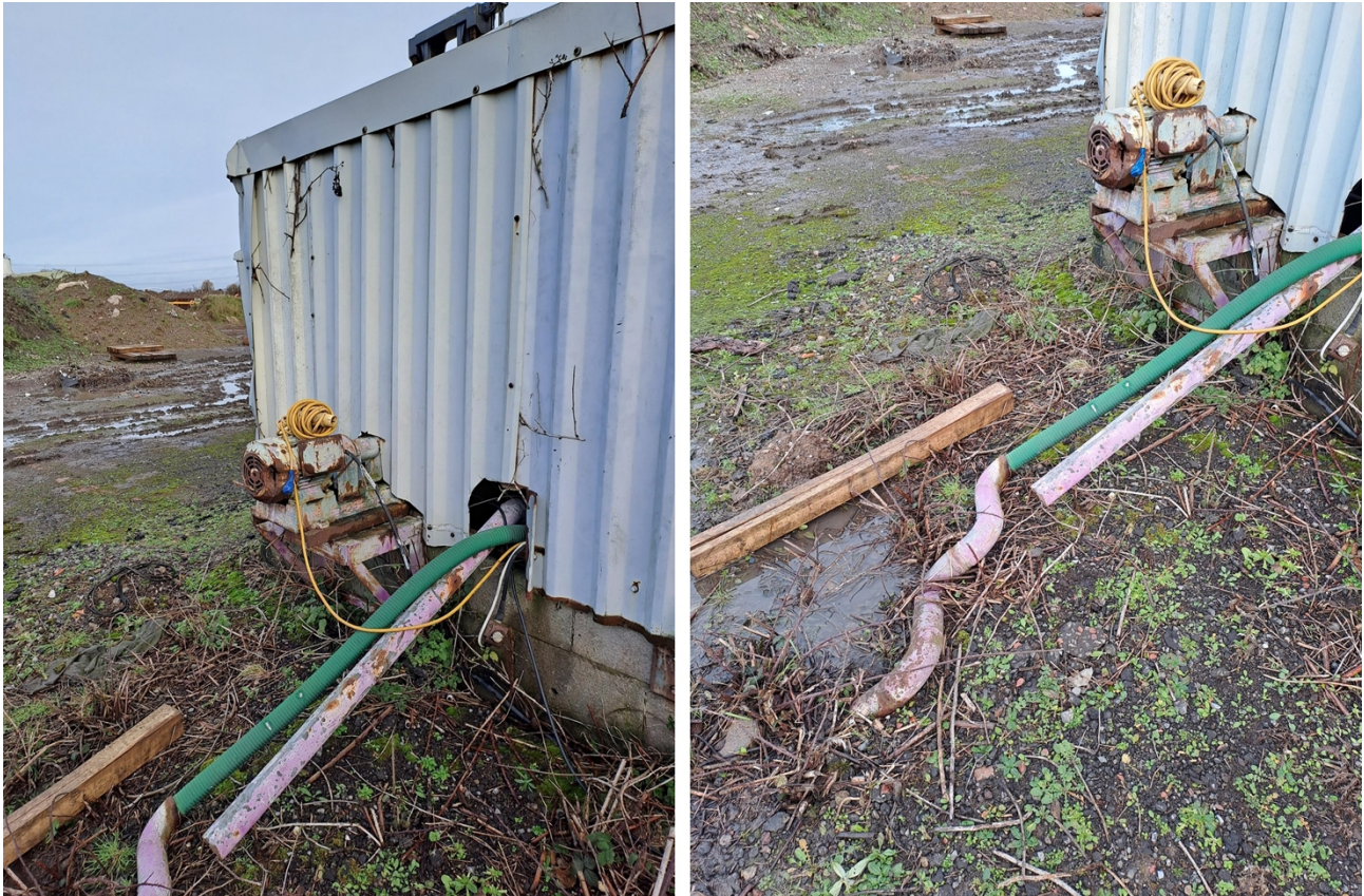
Figure 3 – The rear of the sewage treatment system as observed during the visit.
