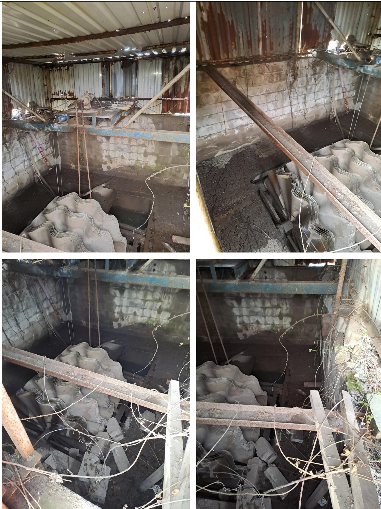
Figure 2 – The condition of the sewage treatment system as observed during the visit.
