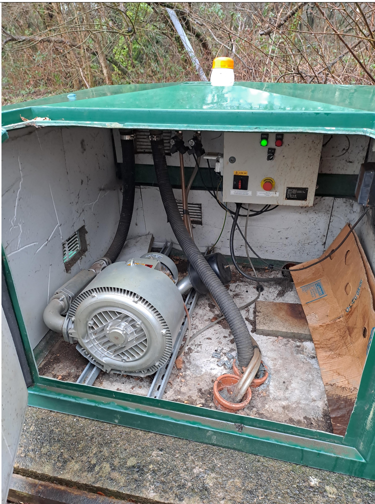
Figure 2 – The alarm and control box as observed during the visit.
