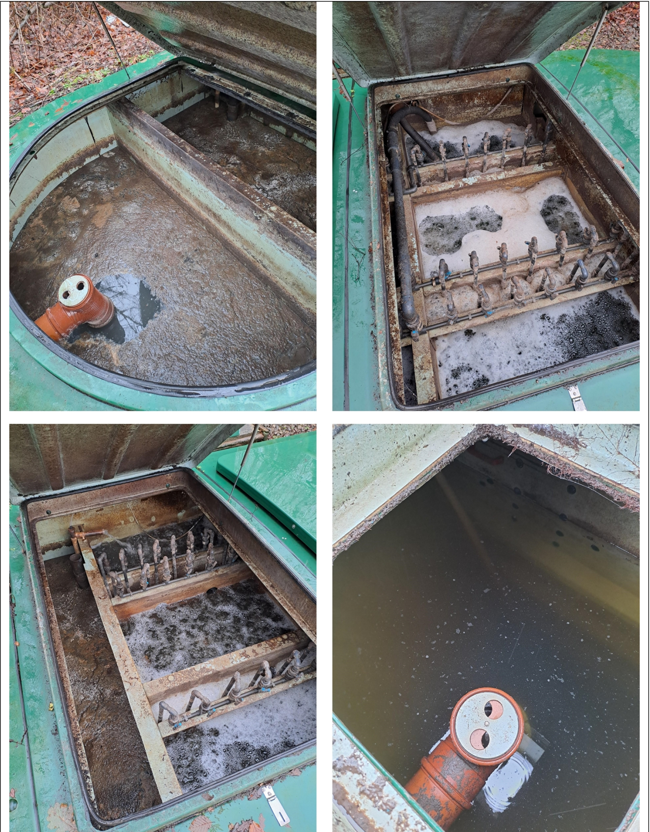
Figure 3 – The treatment system as observed during the visit. From top to bottom, left to right: Primary settlement tank, aeration chamber (1), aeration chamber (2) and final effluent tank.
