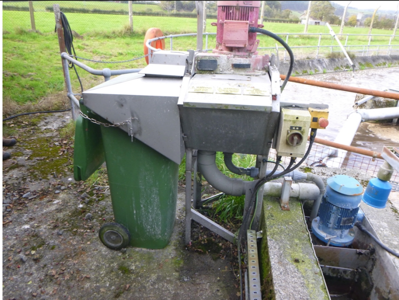
Photograph 3: Screenings deposited into skip/bin
