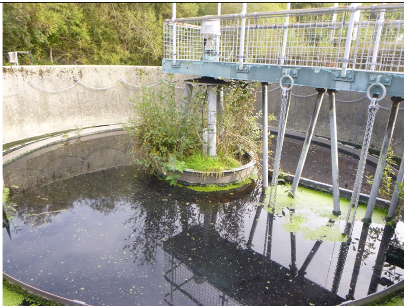
Photograph 7: Final settlement tank
