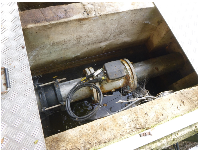
Photograph 8: MCERTS flow meter
