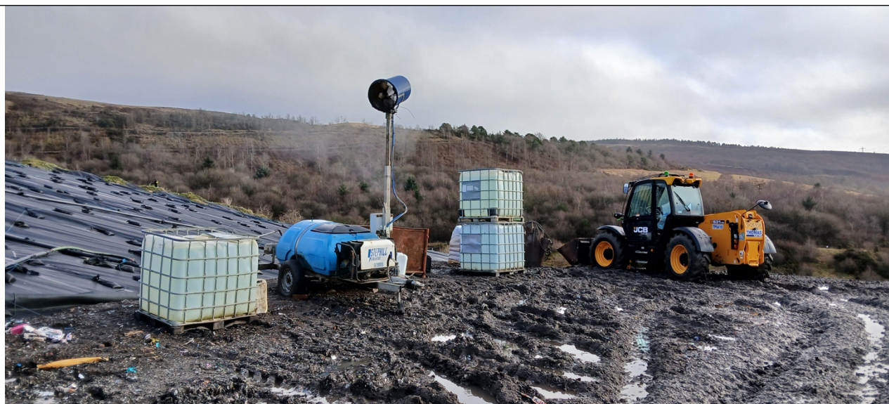
Photo 1 - Odour mitigation measures on site during landfill gas well drilling activities on 28/01/26
