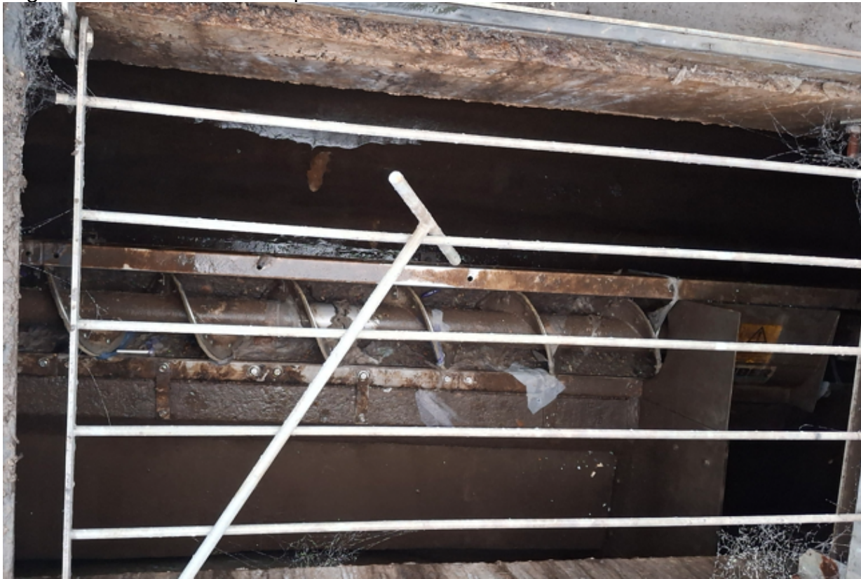
Photo 1: Screws and screen. Rag present overtopping the screen.
