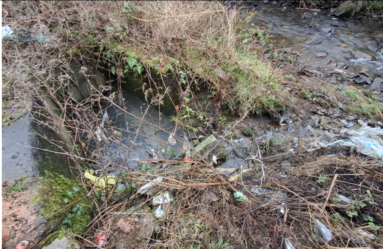
Photo 2: Sewage related debris on apron and surrounding vegetation.
