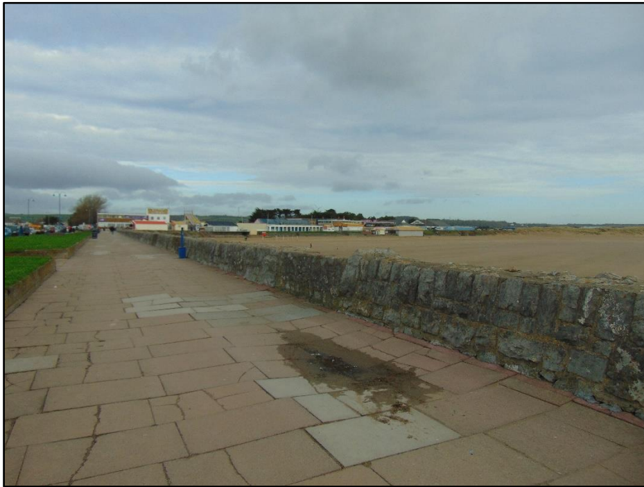
Plate 21. Eastern Promenade: the promenade showing variations/blocked openings in the wall parapet
