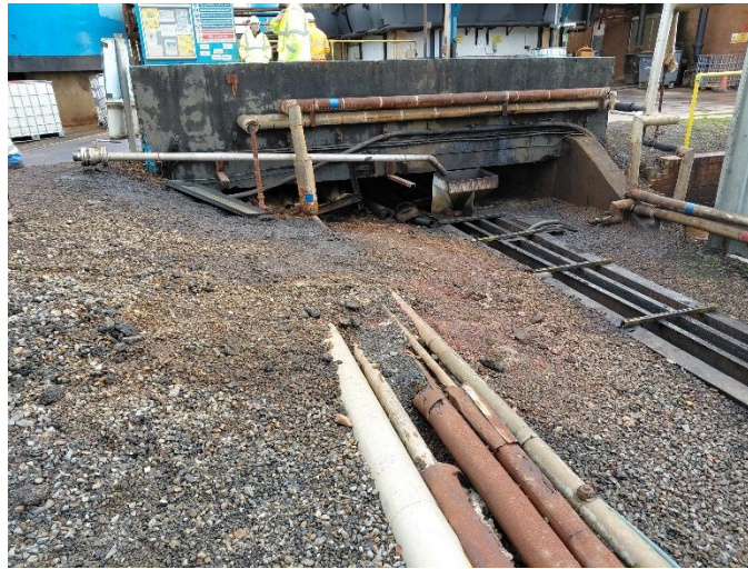
Image 4 corroded and partially buried pipework
