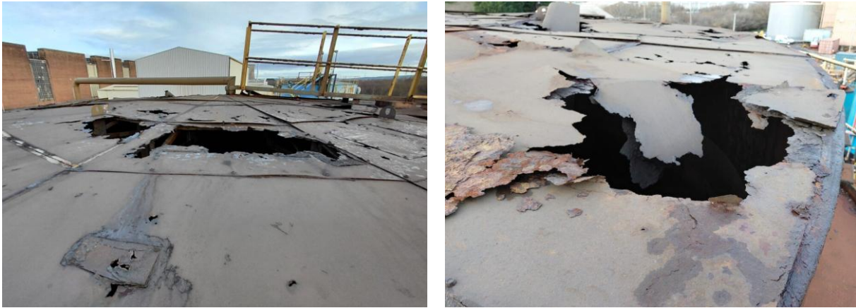
Images 5 & 6 – corrosion on tank roofs
