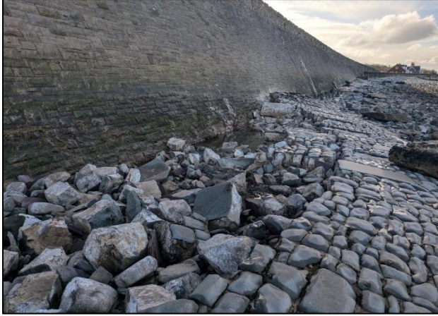
Figure 7: Image of main failure.
