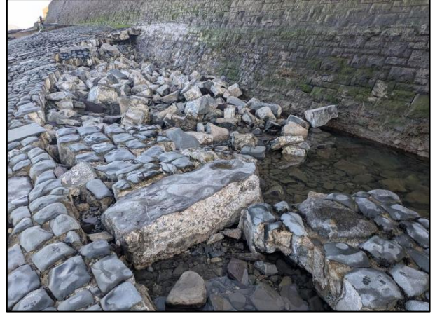
Figure 8: View within failure.
