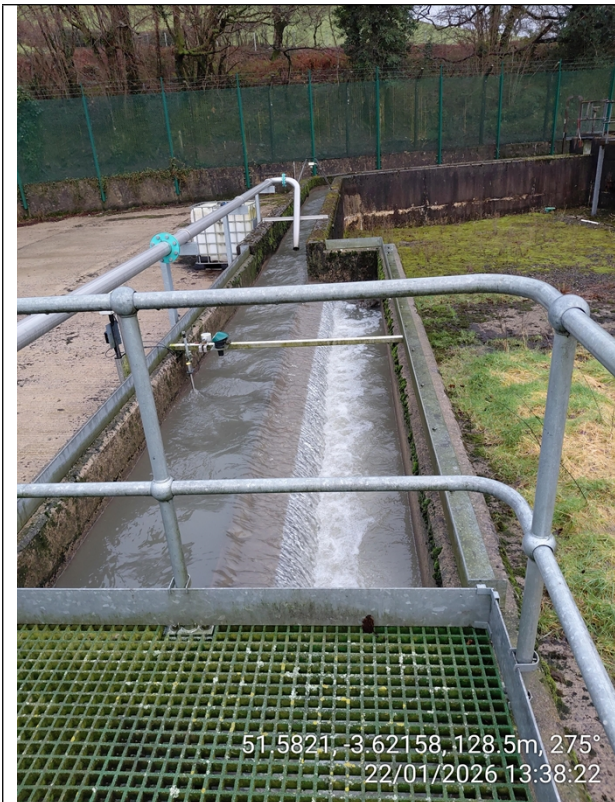
Image 1: Works spilling to storm channel via storm weir
