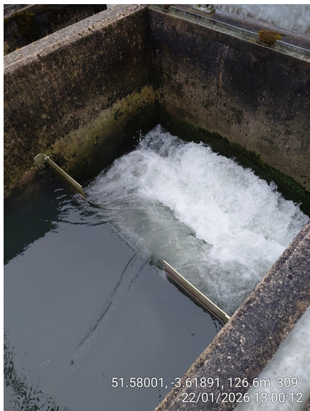
Image 3: Final effluent at monitoring point
