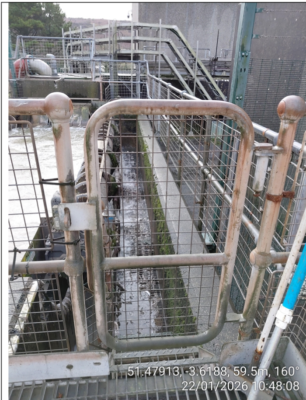
Image 1: Influent spilling to storm channel
