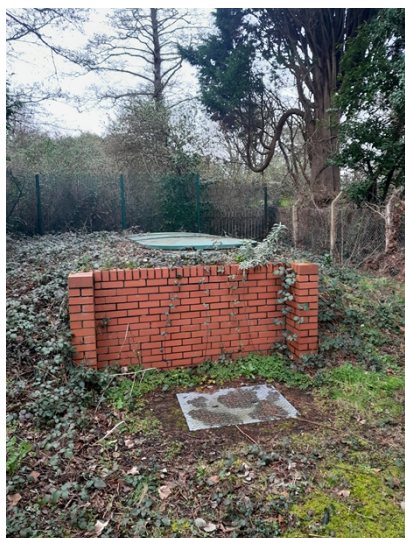
Fig 1 Sewage Treatment Plant
