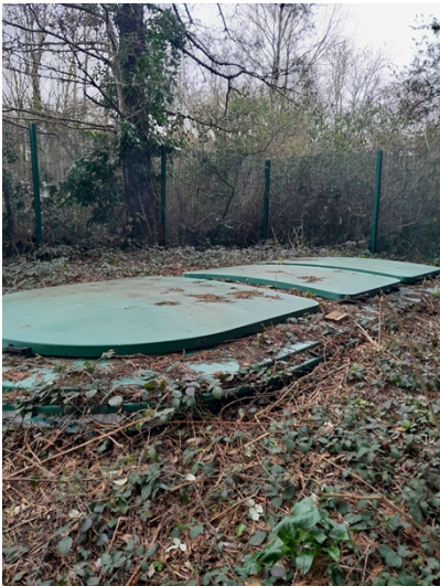
Fig 3 Sewage Treatment Plant
