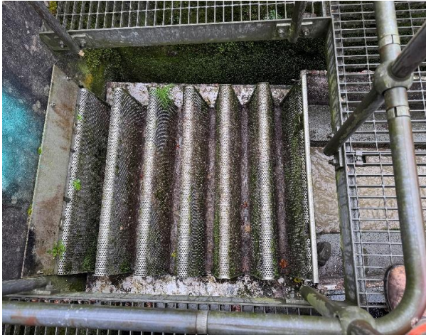
Storm Weir (through wave screen)
