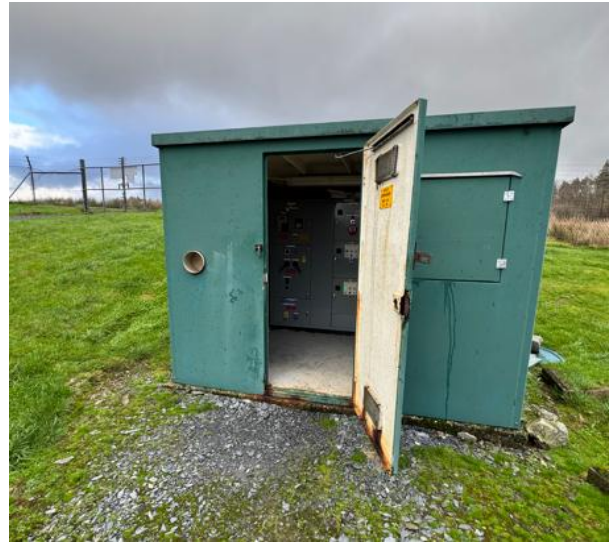
Kiosk where Level Monitor Display is Located
