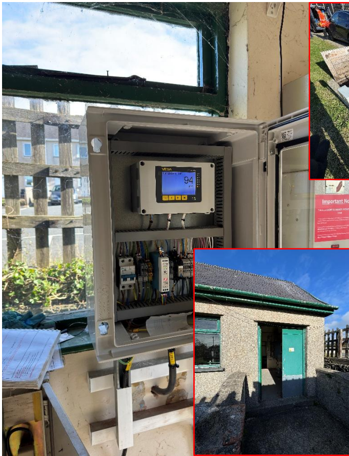
Level Meter Location.
