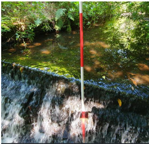
Extra Feature (old weir, this is from former waterwheel at Plas Cilybebyll) Weir visible in upstream photo above as well). Weir is about 2.5m high.
