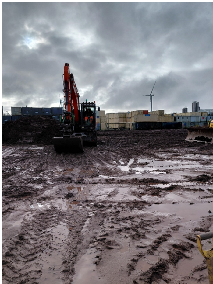
Photo 2. Water logged ground after period of prolonged rain.
