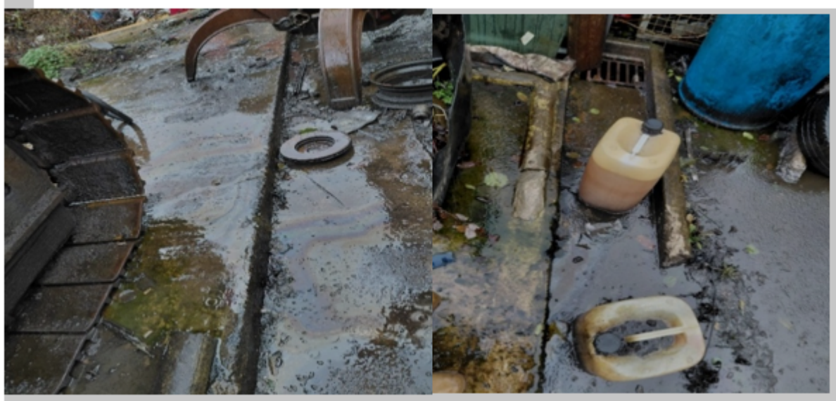
Photos 1 & 2 showing the raised pavement damaged on inspection on Nov 25
