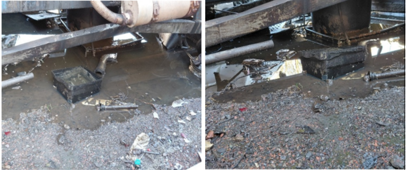
Photos 5 & 6 showing drip tray on inspection on Feb 26
