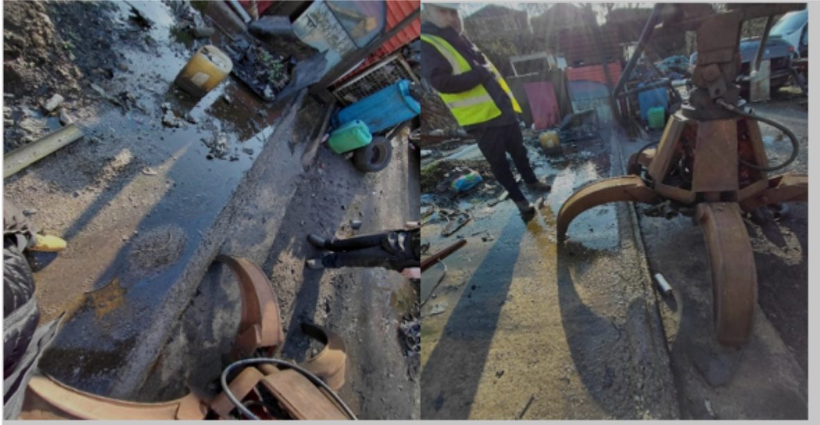
Photos 3 & 4 showing the raised pavement now repaired on Feb 26
