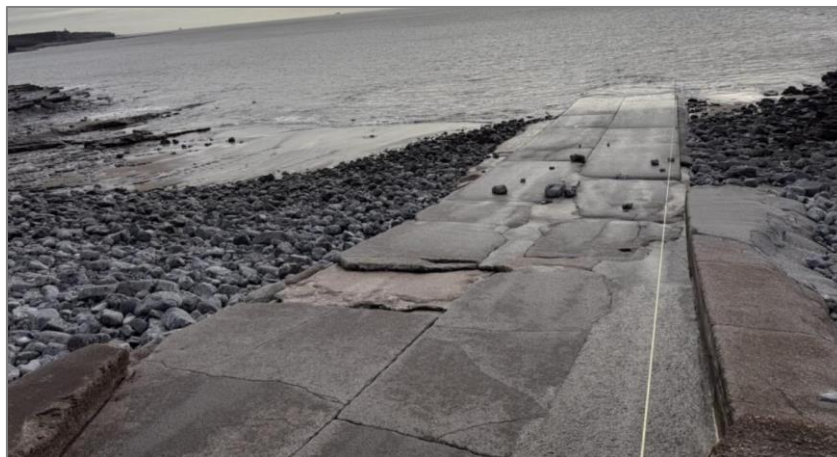
Figure 1: Photo of damage to upper-level ramp of slipway
