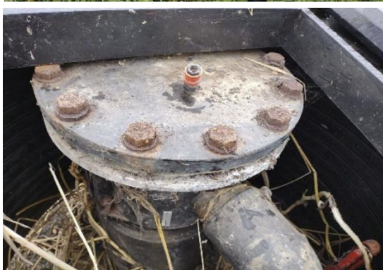
LW12 – top plate / gasket, damaged Tefen valve
