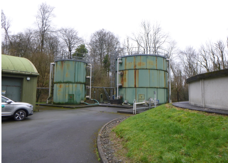
Photograph 4: Sludge holding tanks
