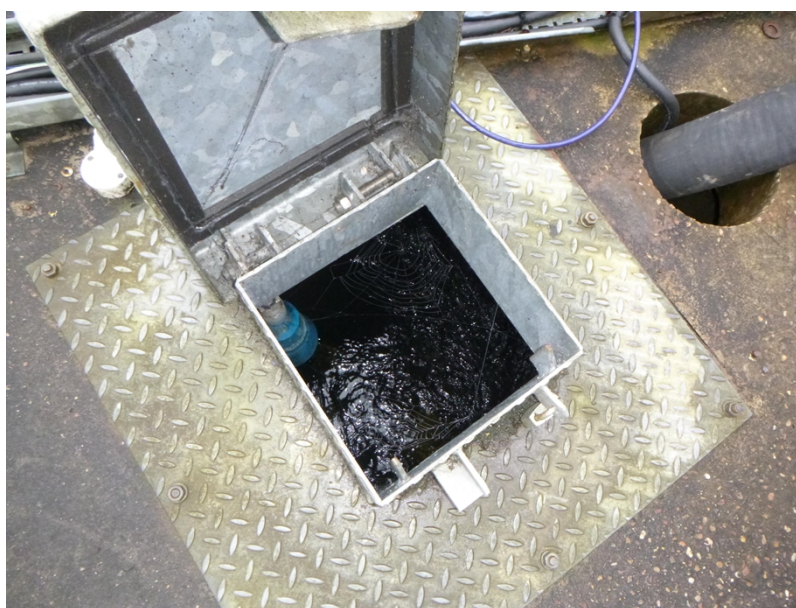
Photograph 6: Final effluent sampling point
