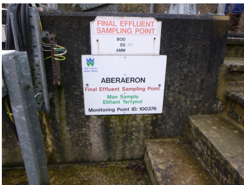
Photograph 5: Final effluent sampling point signage
