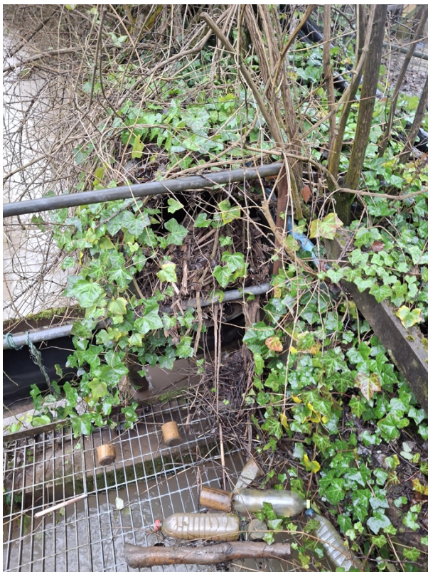
Figure 1: No discharge from storm overflow
