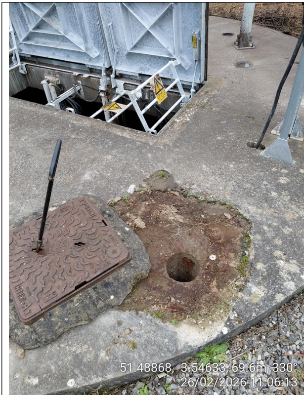
Image 1: potential overflow location
